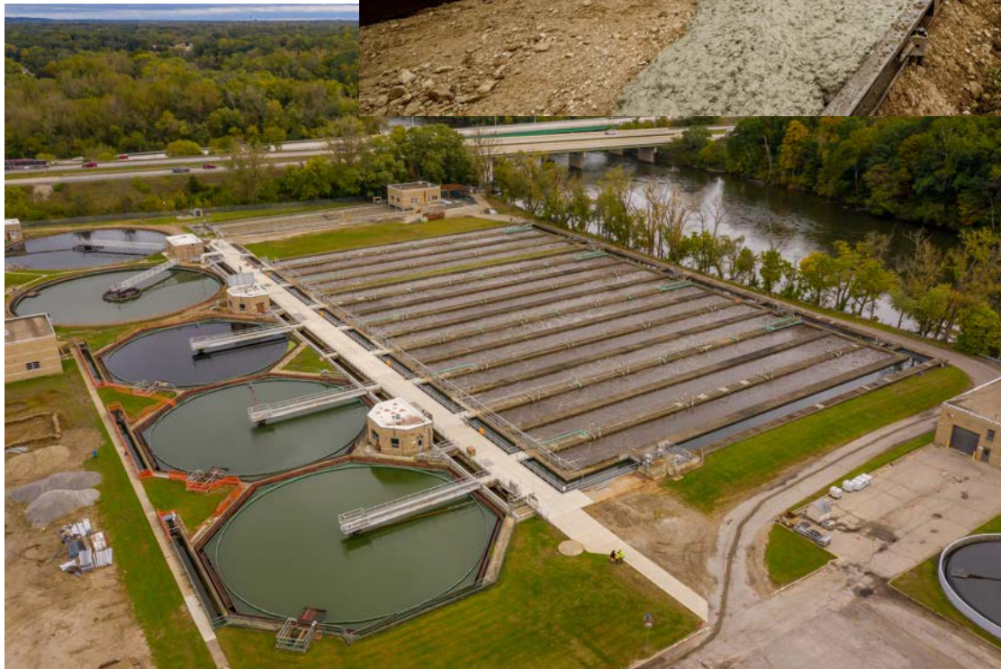
Wastewater Treatment Plant
