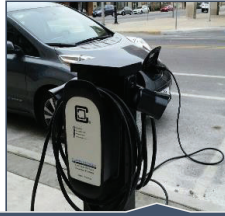
Electric Vehicle Charging
