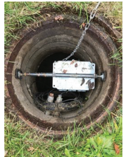
Smart Sewer Sensor
