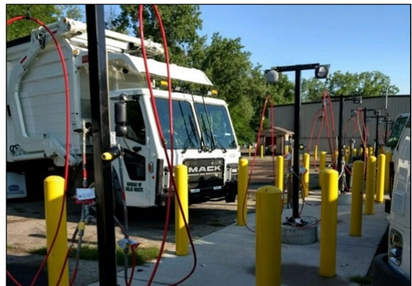
CNG Fill Station at the Riverside Drive location
