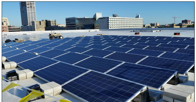
Century Center Solar Panel Roof
