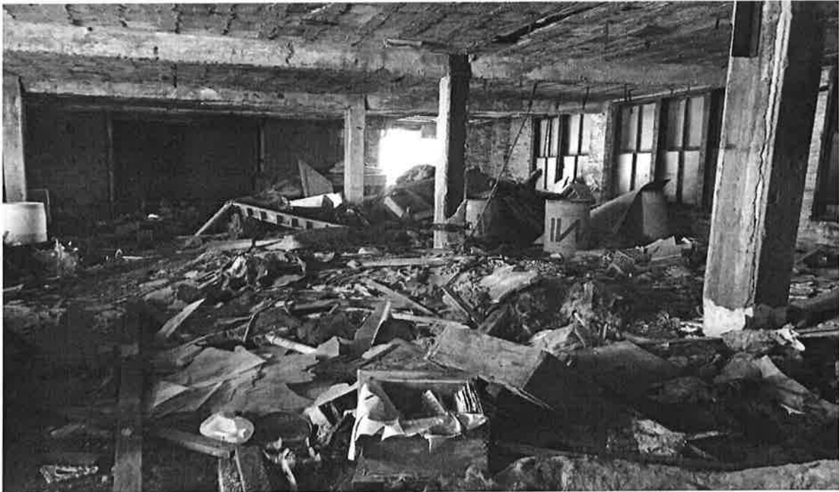
Photo 4: Drums inside building under debris
