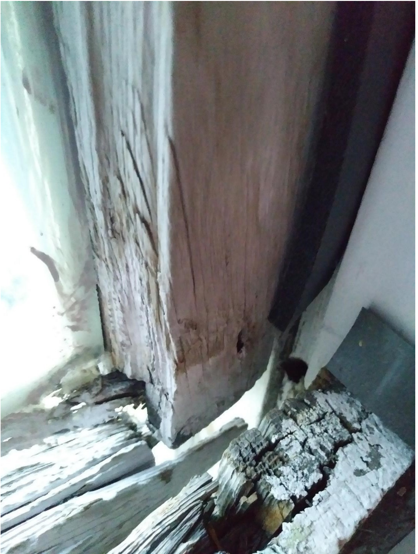
Figure 5 - Applicant supplied image of the deteriorated sash.
