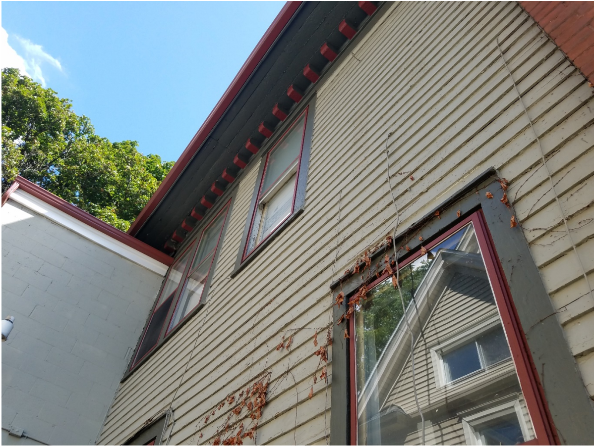
Figure 10 - North face, upper three windows to be replaced.
