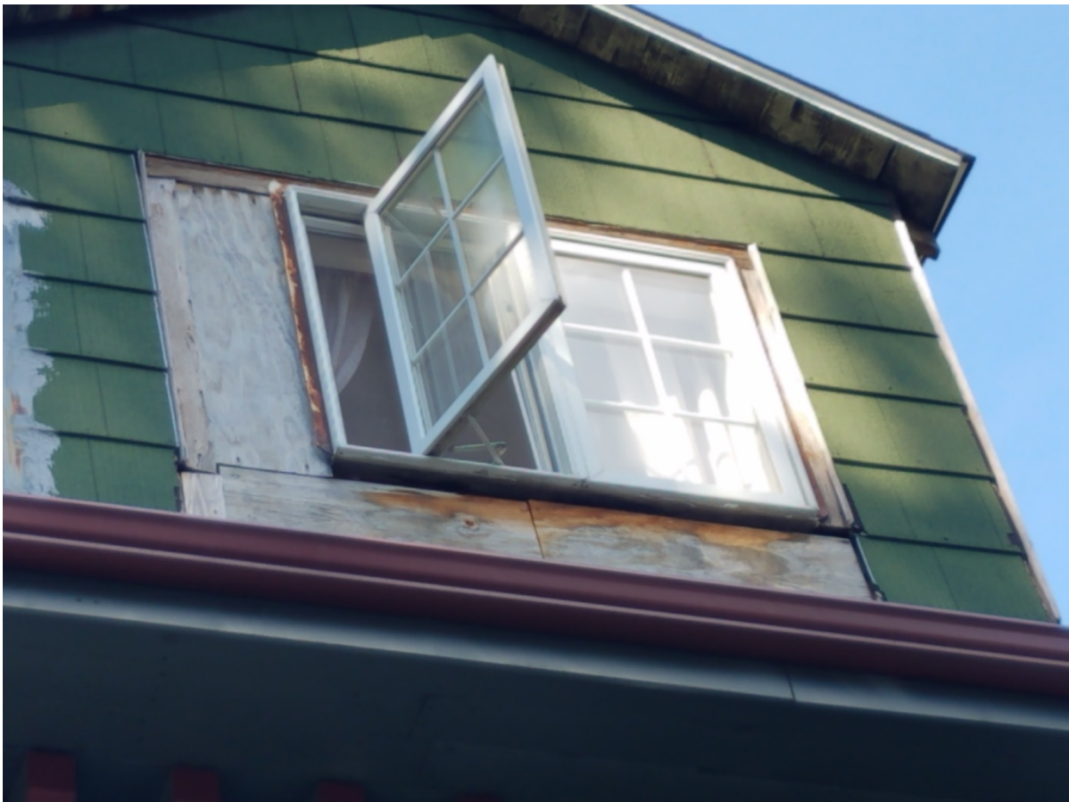
Figure 17 - Close-up of ill-fitting window and mastic siding.
