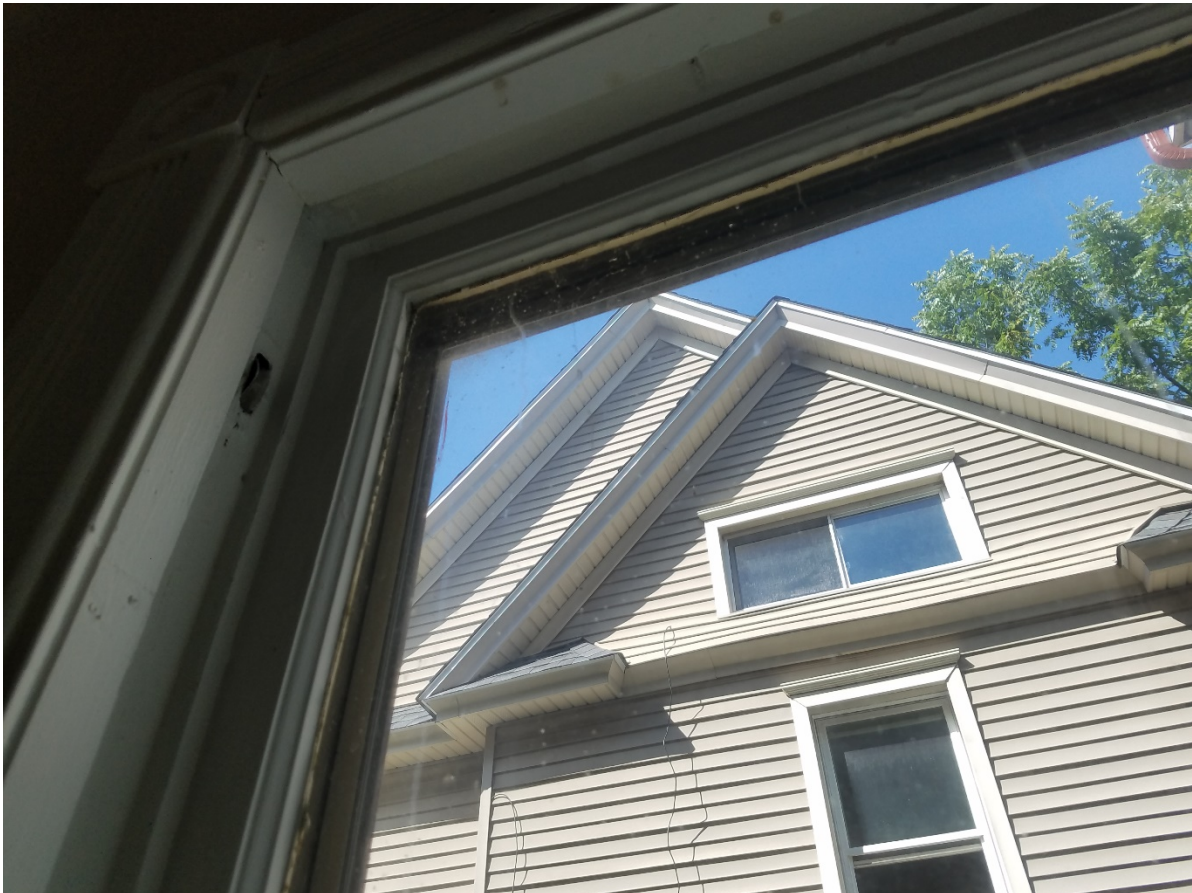
Figure 13 - Missing weights / ropes.
