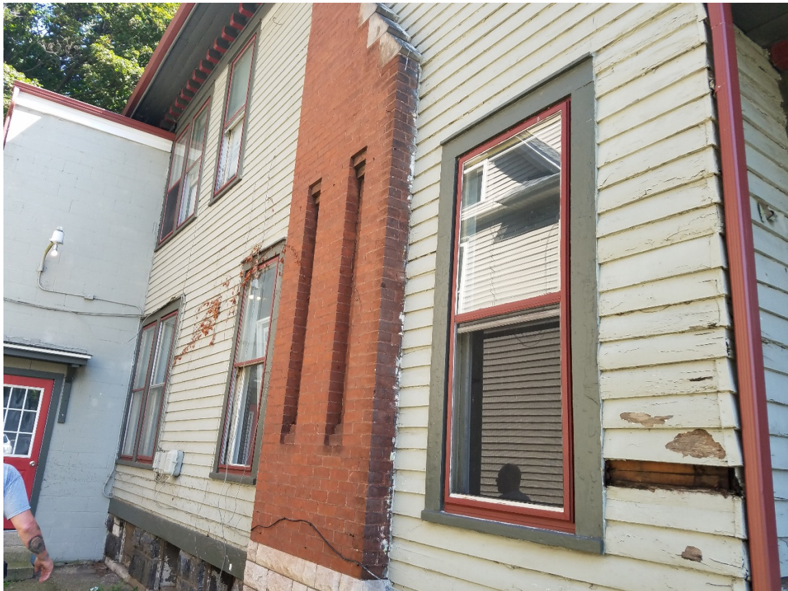
Figure 11 - North face, all windows to be replaced.
