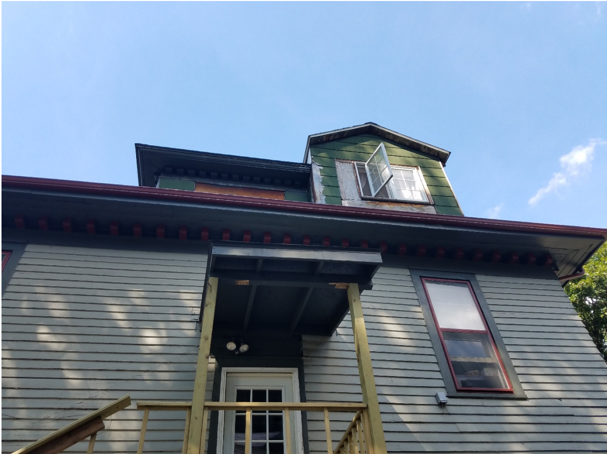
Figure 16 - South gable with window (replaced by previous owner without COA), mastic/asphalt siding.
