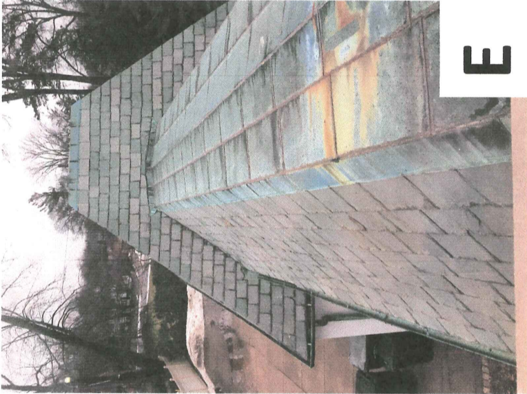
EXISTING CONDITIONS PHOTO - E ELECTRICAL SECOND FLOOR WINDOW LOOKING SOUTH EAST DOWN AT PROPOSED LOCATION FOR THE FAMILY ROOM ADDITION
