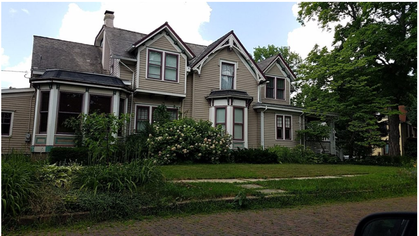
Figure 3 -- 801 Park, looking north from Manitou Place. Main chimney visible at left, while the subject chimney is obscured by the roof line.
