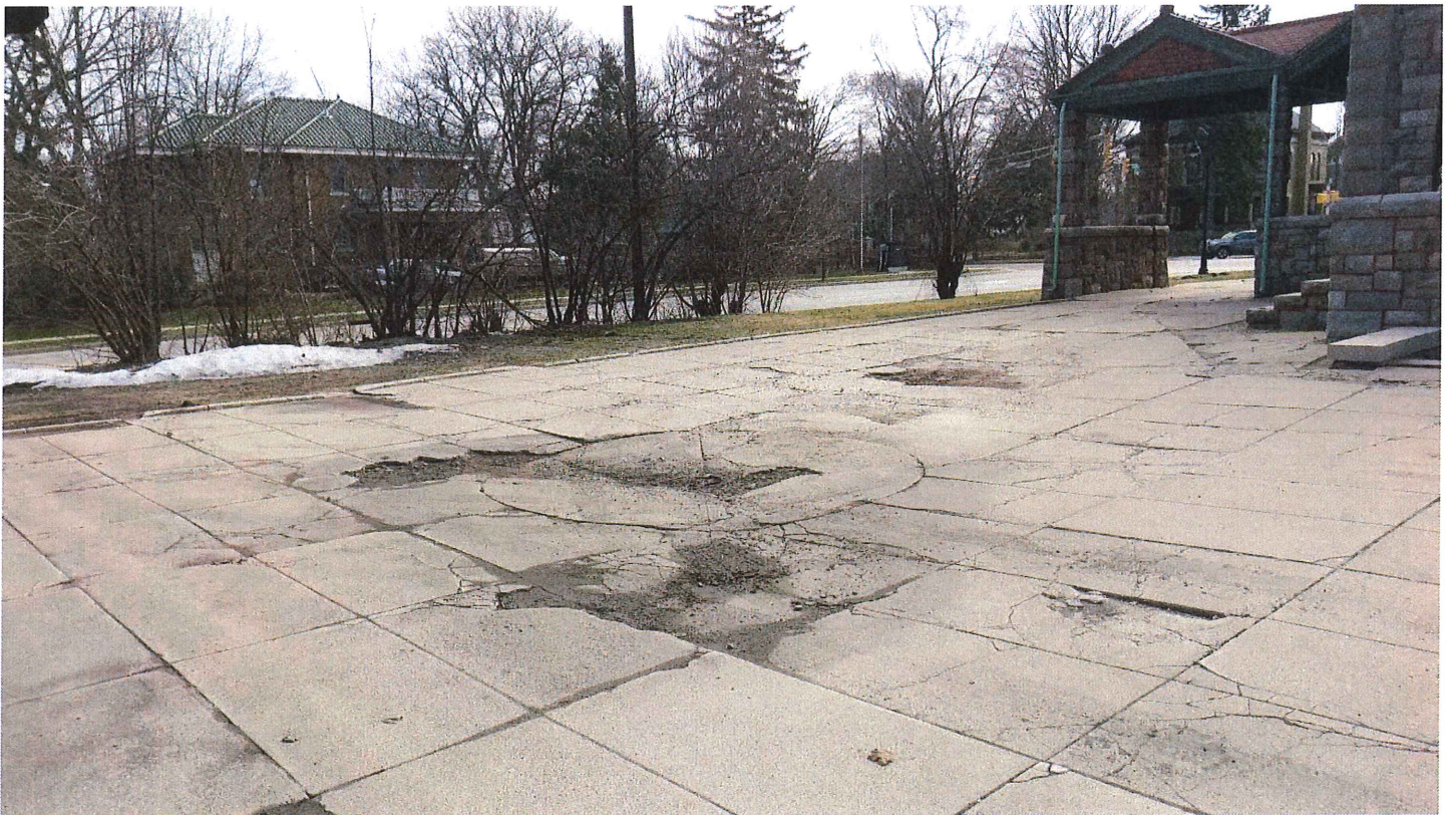
Concrete is crumbling and uneven/missing
