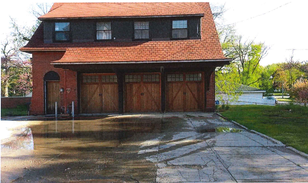
Drainage issues – water pools, comes up to the entrance and overhead doors before draining down west side of building
