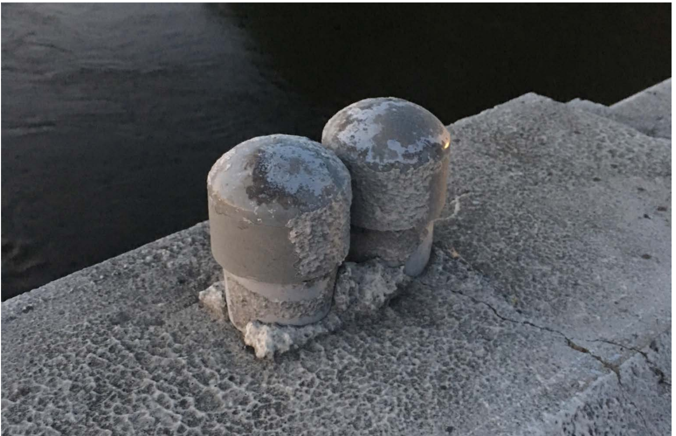
Figure 2 - Existing conduit, with caps. New pole to be installed atop this location.
