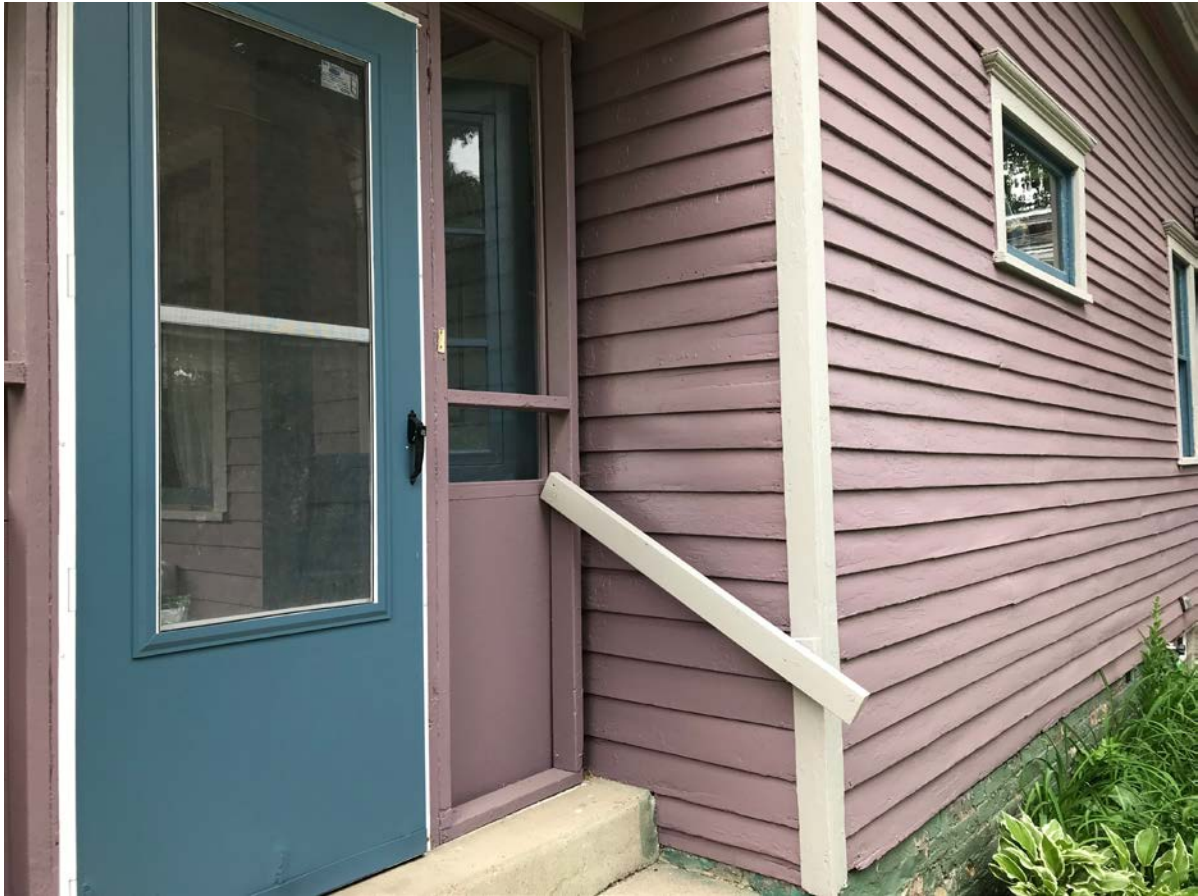
Figure 3 - South east face. Entrance screened-in porch at left. Railing to be replaced at center.
