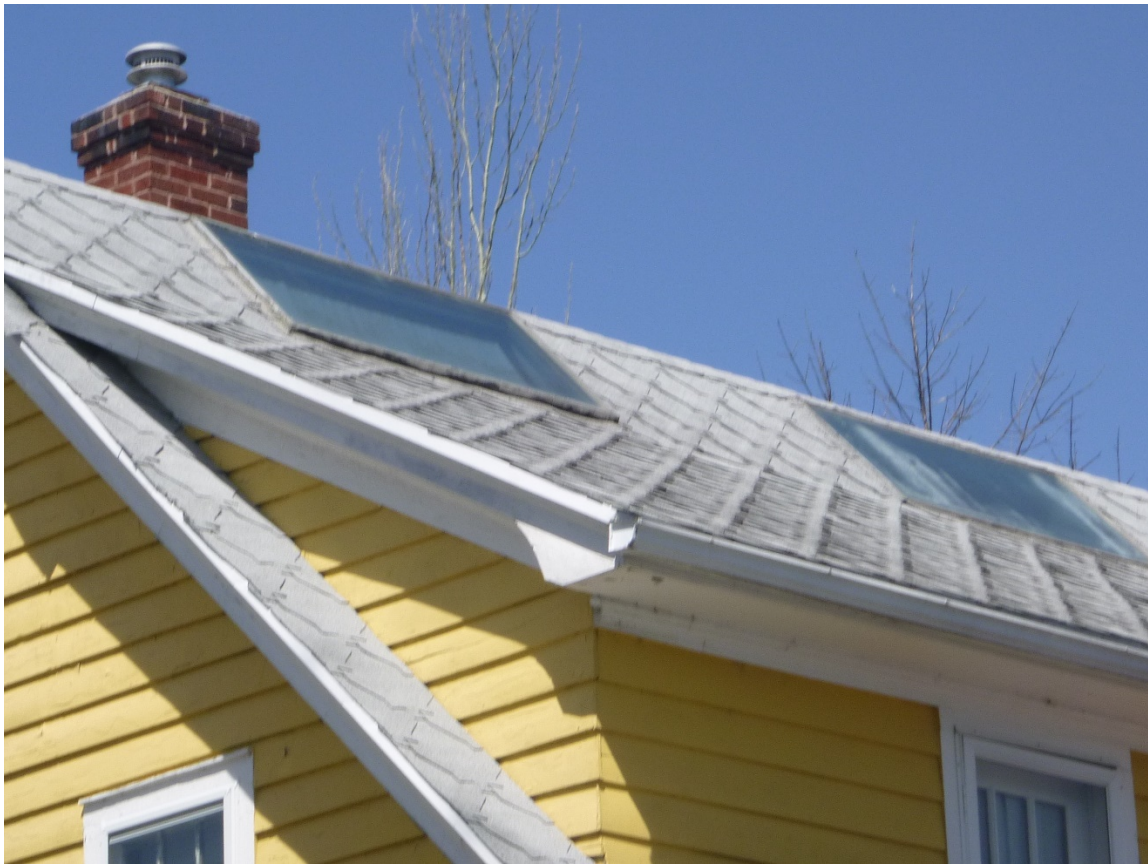
Figure 2 - Skylight condition, April 30, 2018
