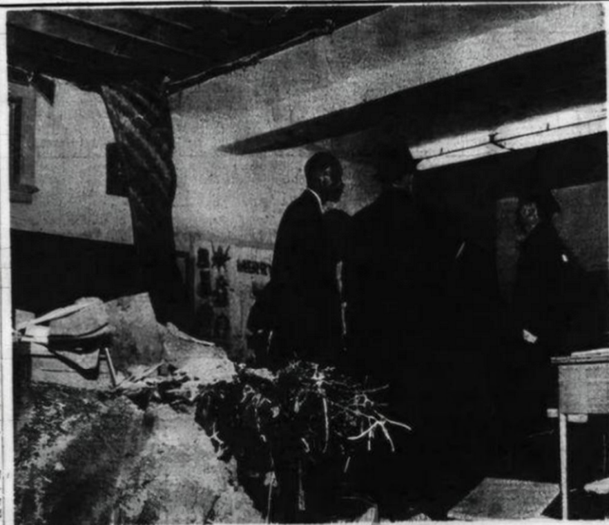
LINDEN SCHOOL, CEILING FALLS — A Christmas tree lies buried beneath debris on the teacher's desk as Principal Edward Myers, left foreground, and Fire Chief Cecil McHenry discuss the possible cause of a ceiling collapse this morning in a basement third grade classroom at Linden School.
