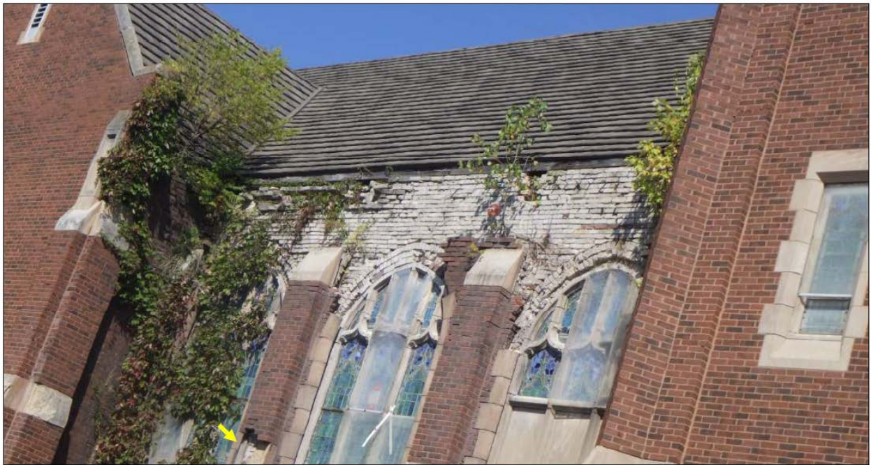
Photo 9: Collapsed outer wythe of brick on the south elevation of the sanctuary wing. Note the vegetation growth and deterioration in the buttresses (arrow).
