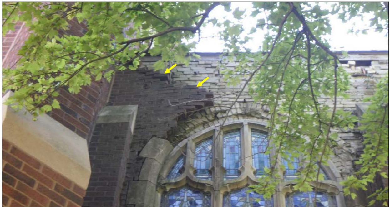
Photo 10: Collapsed outer wythe of brick on the south elevation of the sanctuary wing. Note the loose bricks with open mortar joints (arrows).
