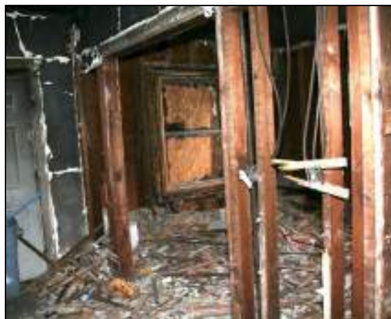
fig. 24 Interior of above dilapidated house
