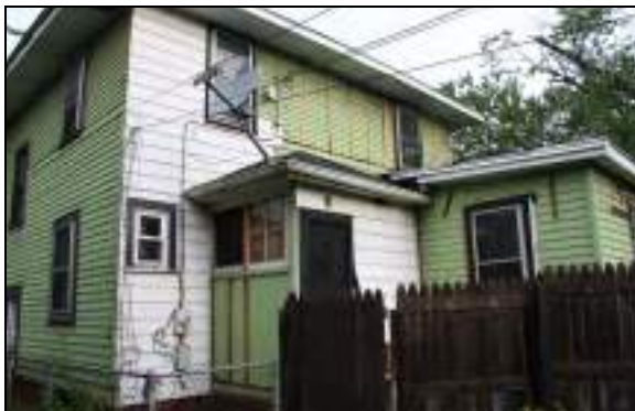
fig. 27 Vacant house that is a candidate for order to repair proceedings
