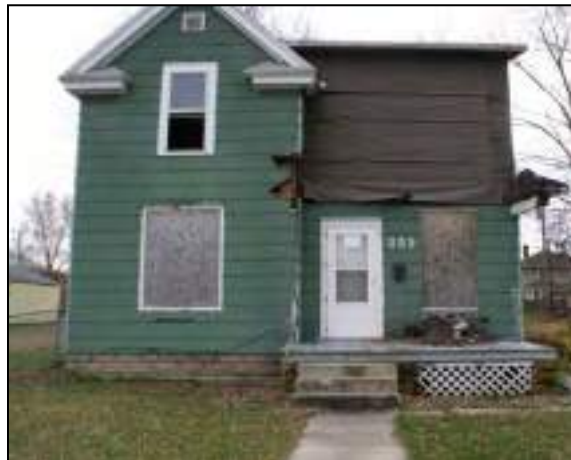
fig. 23 Exterior of a dilapidated home which requires inspection prior to pursuing demolition
