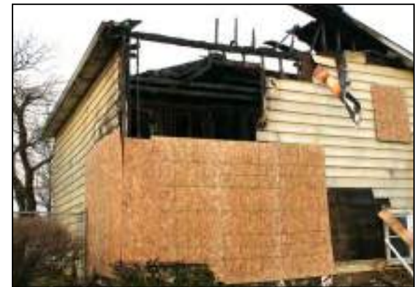
fig. 22 Fire damaged houses are a hazard to the community and are torn down as quickly as possible
