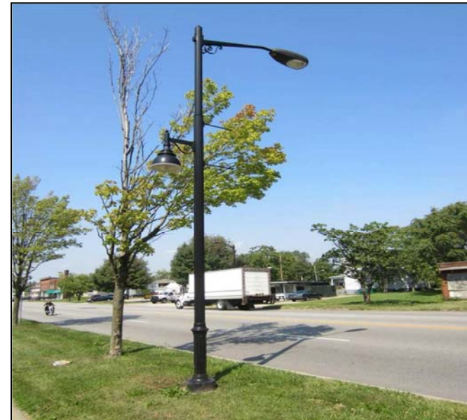
Photo 20 - Existing lighting provides safety and decoration along the Lincoln Way West corridor
