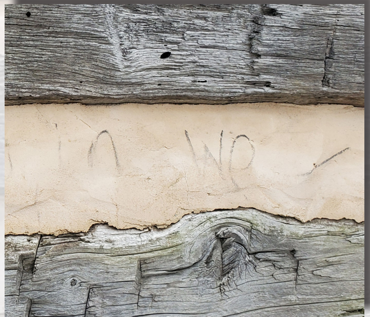
Evidence of graffiti on the cabin
