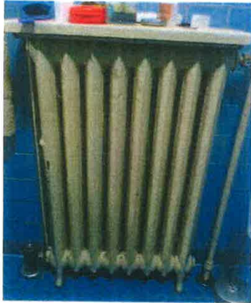
BATHROOM - RADIATOR, SIDE D
