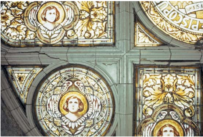
Figure 12. Stained glass frames are typically wood, steel or stone; however, other materials, and their inherent problems, can also be found as seen in this photograph of cracked terra cotta frames from 1926.
