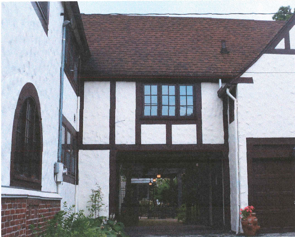
Existing Condition at Pass-Thru
