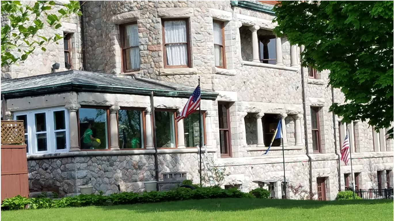
Figure 2 - Rear porch (enclosed) porch area. Non-compliant windows in white at left, replaced (compliant) windows at right. Windows needing restoration visible on the main structure. Photo from May of 2018.
