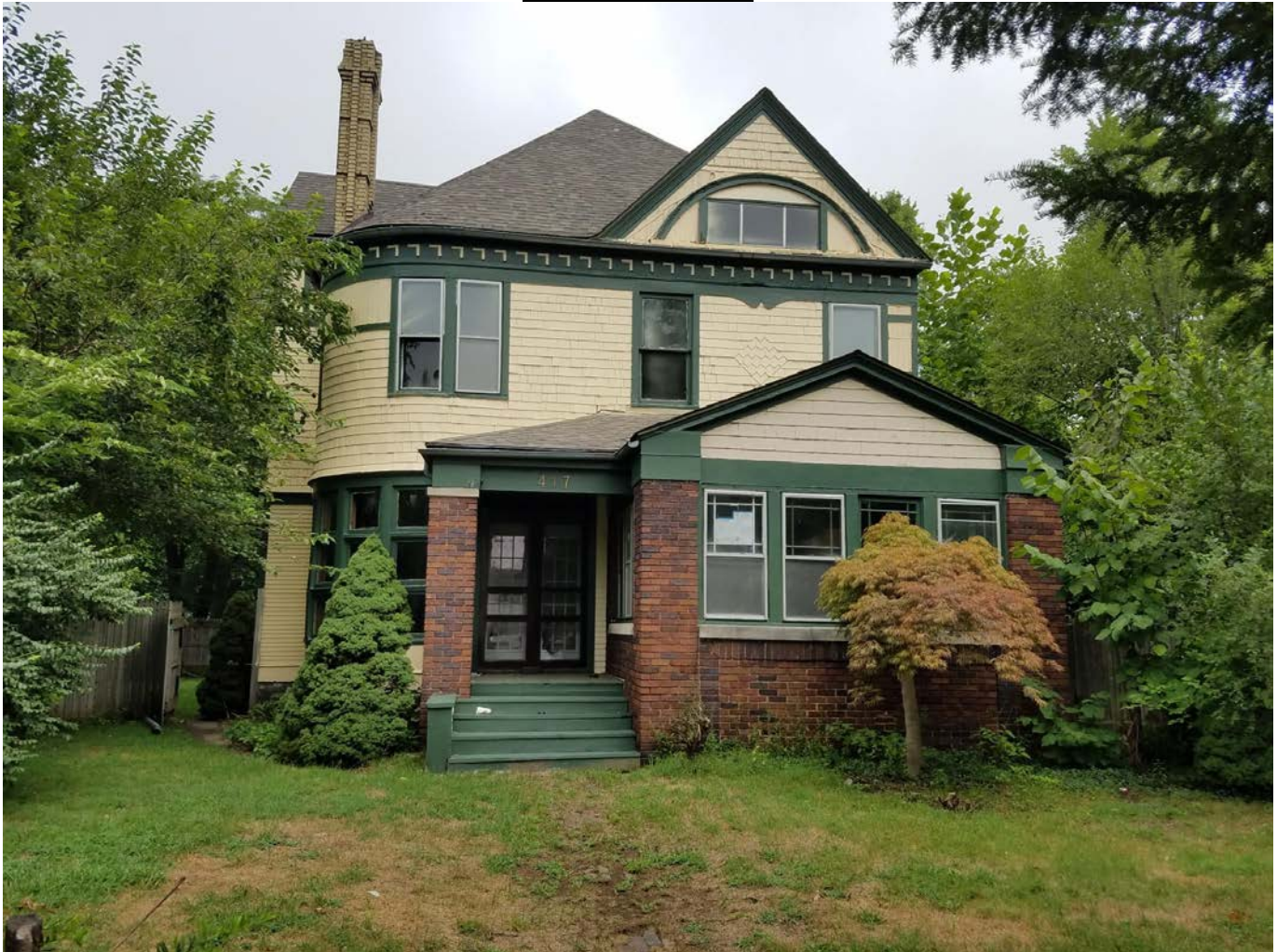
Figure 1 – 417 W Navarre from the street, looking north. The subject door is behind the storm doors.
