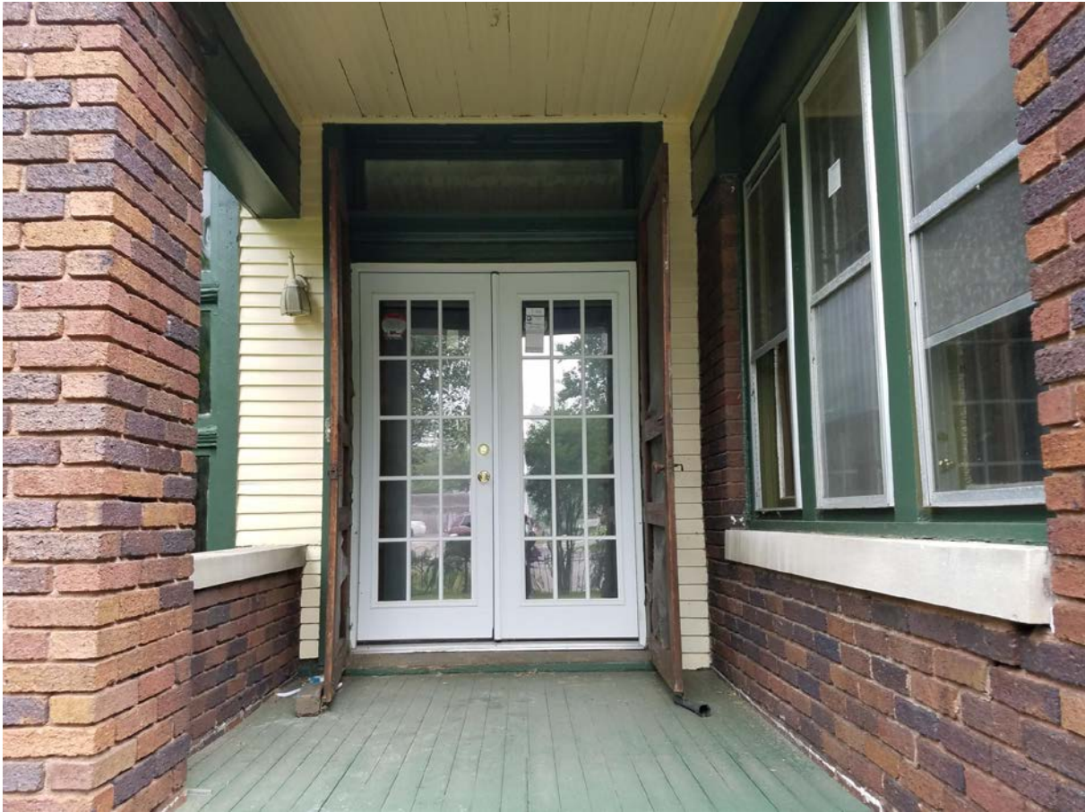
Figure 2 -- Close-up of the replacement doors on the front porch of the structure.
