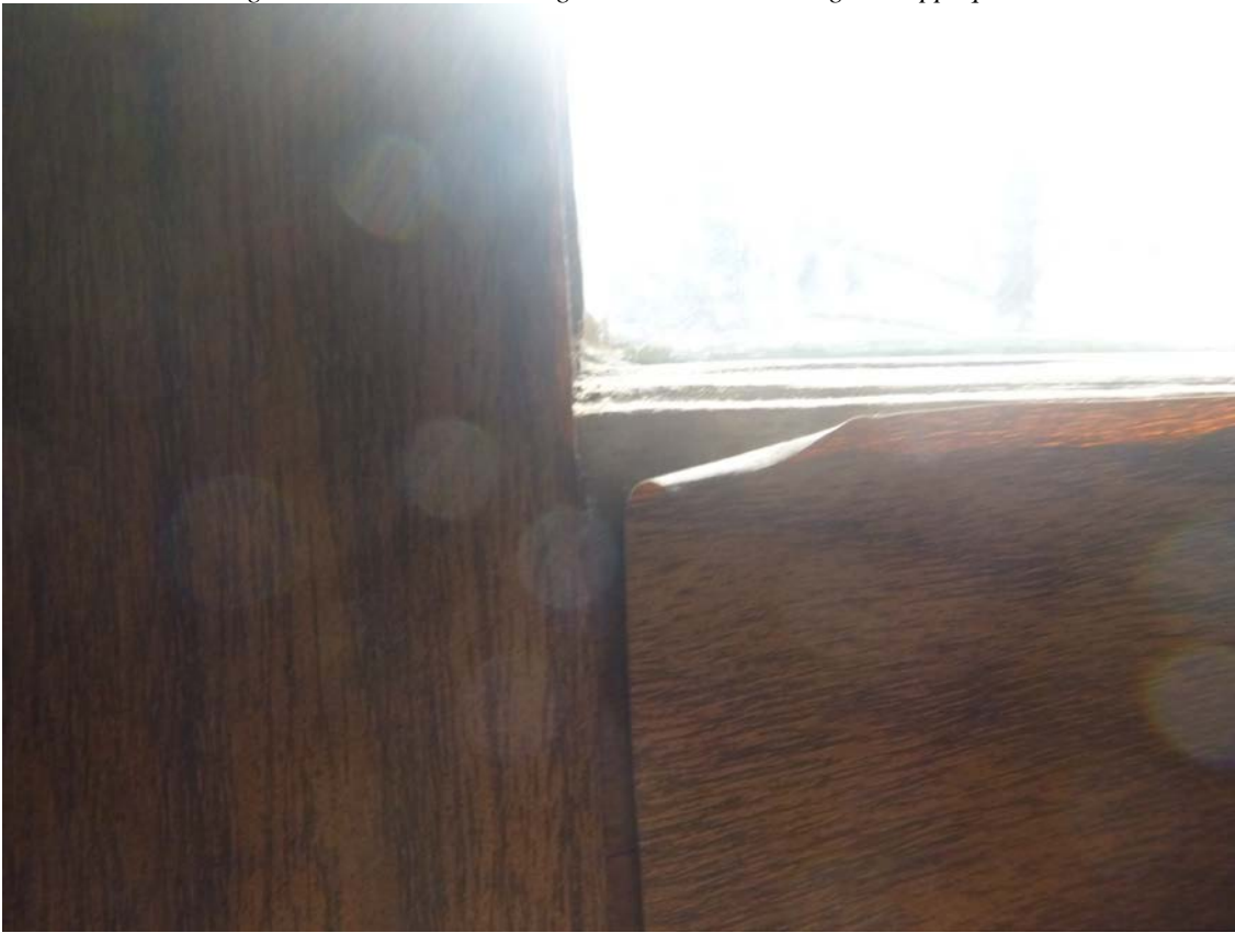
Figure 7 - 608 Park - close-up of peeling applique.
