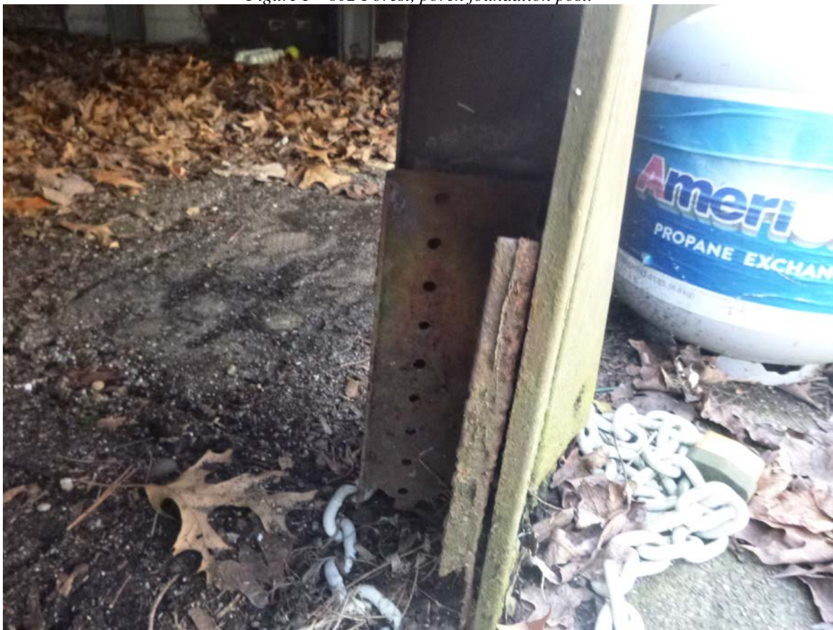
Figure 6 - 802 Forest, degrading porch posts.
