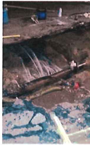
Main water leak
