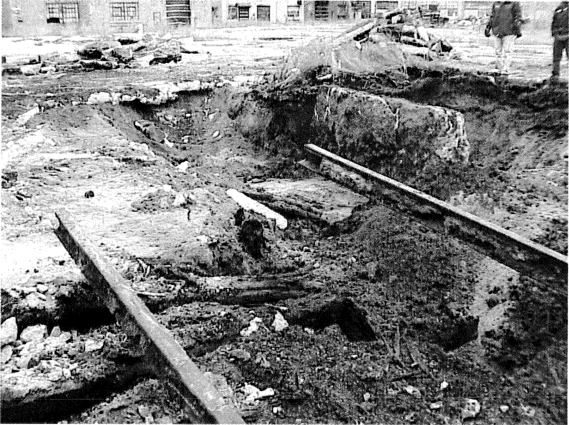
The steel rails and ties of the rail spur are imbedded in the concrete. This view is looking northeast toward the north end of the excavation. One of the concrete monoliths is visible above the rail on the right. The petroleum impacted soil is dark gray and dark grayish brown.
