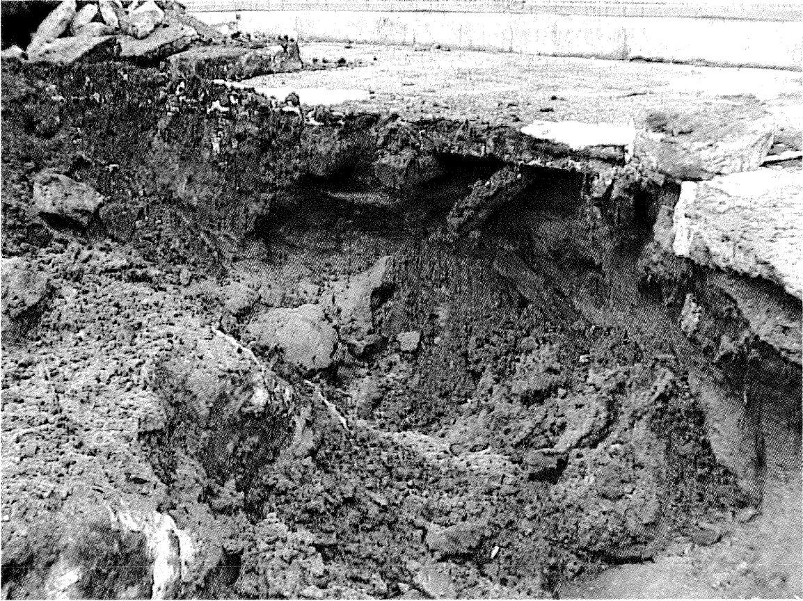
This view is of the west wall of the excavation as impacted soil is being progressively removed to the foundation of Building 93 in the background. The impacted soil is the distinct dark grayish brown material exposed in the wall and bottom of the excavation.
