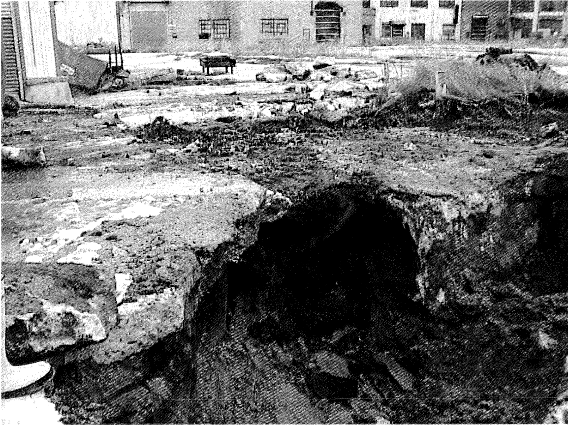
This photograph was taken at the beginning of the excavation of the impacted soil near the center of Area A. Visible is discolored, petroleum impacted soil, one of the buried metal pipes in place, and the first of the concrete monoliths encountered in the excavation area. The view is looking toward the northeast.
