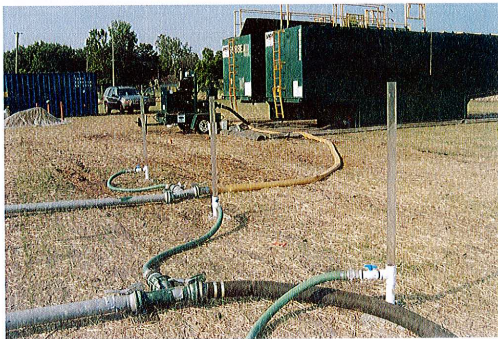
No. 6 – This photograph illustrates the main feed from the mixing/injection pump to the well field distribution system.
