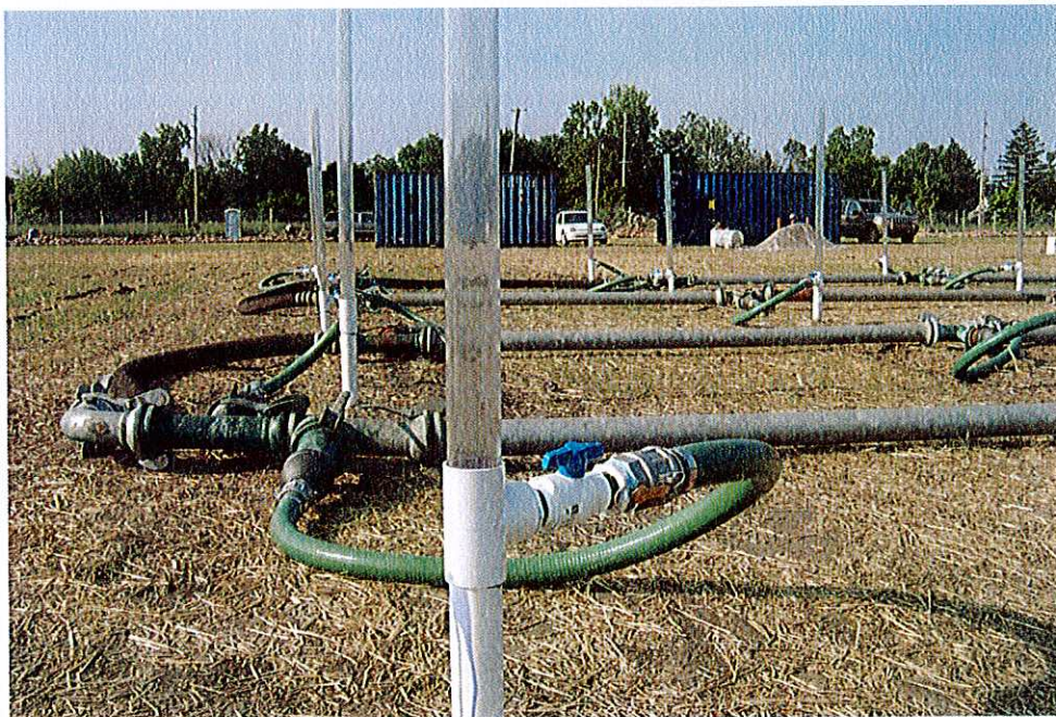
No. 5 – This close up image illustrates a typical injection well head and its control valve.
