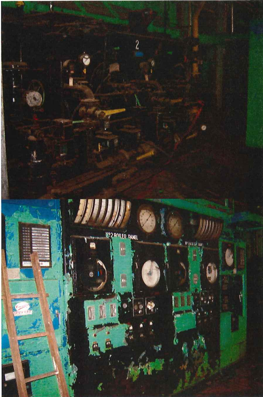
Boiler #2 located in power plant building.
