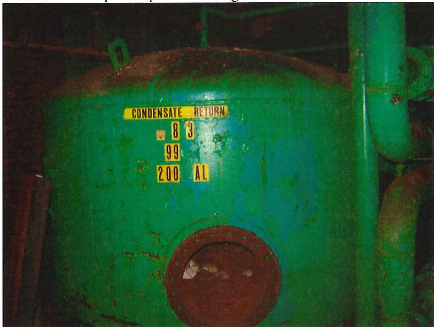
Aboveground process/treatment tank used in power plant building.
