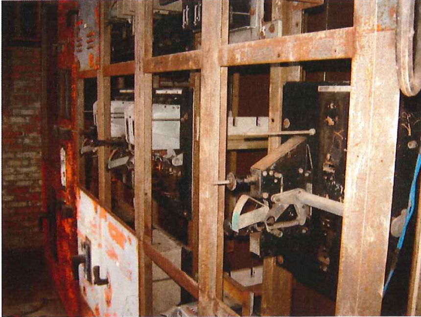
Electrical console equipment (relays, switches, etc.) inside power plant building.
