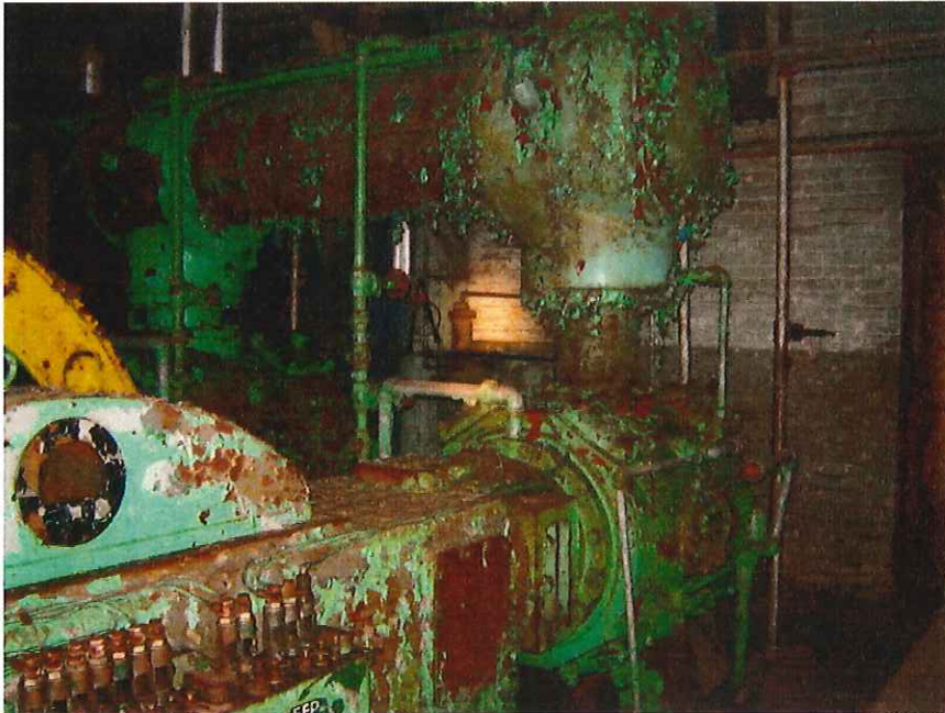
Additional photo of air compressor equipment.
