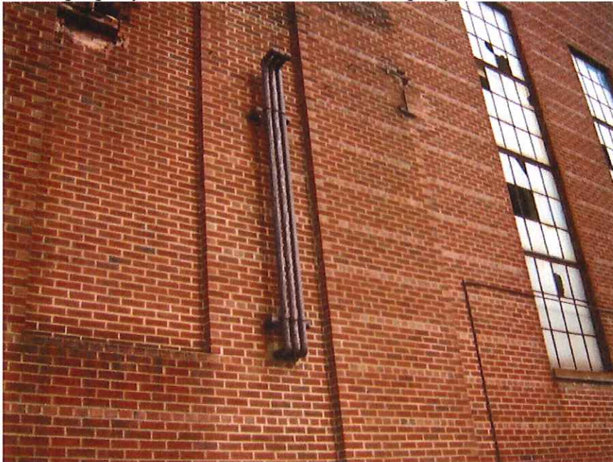
Possible vent lines associated with the hot water boilers.
