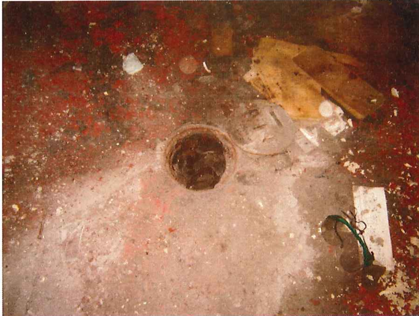
Floor drain inside power plant building.
