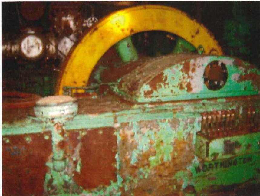
Worthington steam-powered air compressor.
