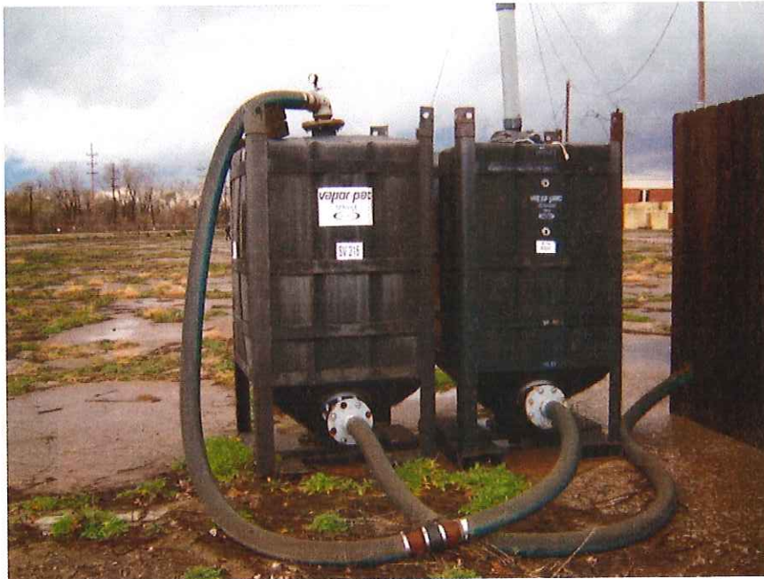
Activated carbon units used to filter and treat impacted groundwater.
