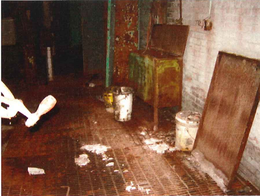
Interior of power plant building, white material is asbestos.
