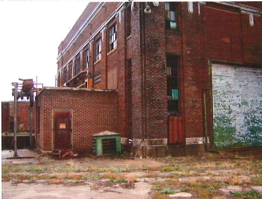
Electrical substation located near southwest corner of power plant building.
