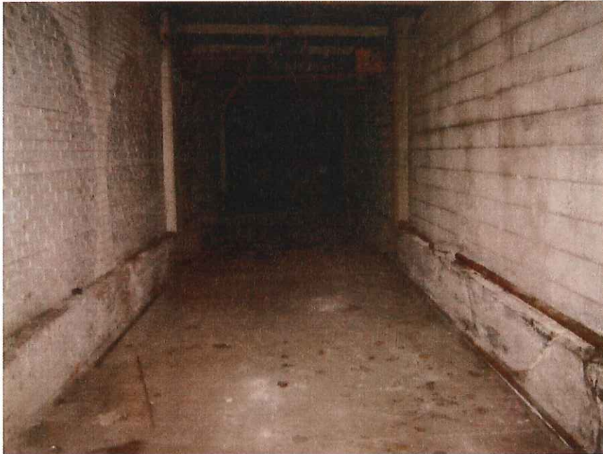
Corridor inside power plant building.
