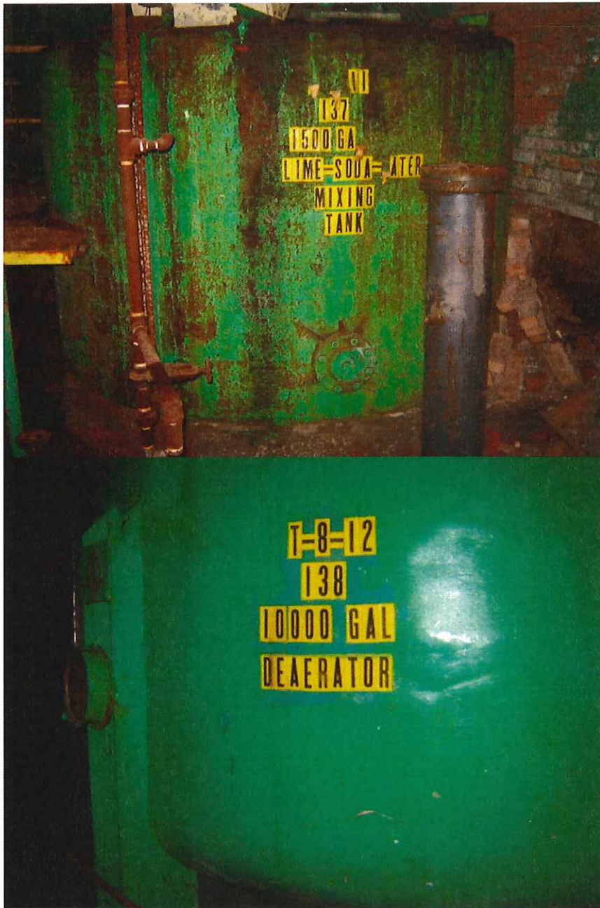
Additional aboveground process/treatment tanks.
