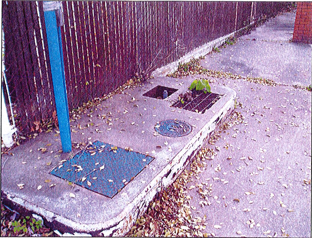
Additional UST system - former diesel dispenser island
