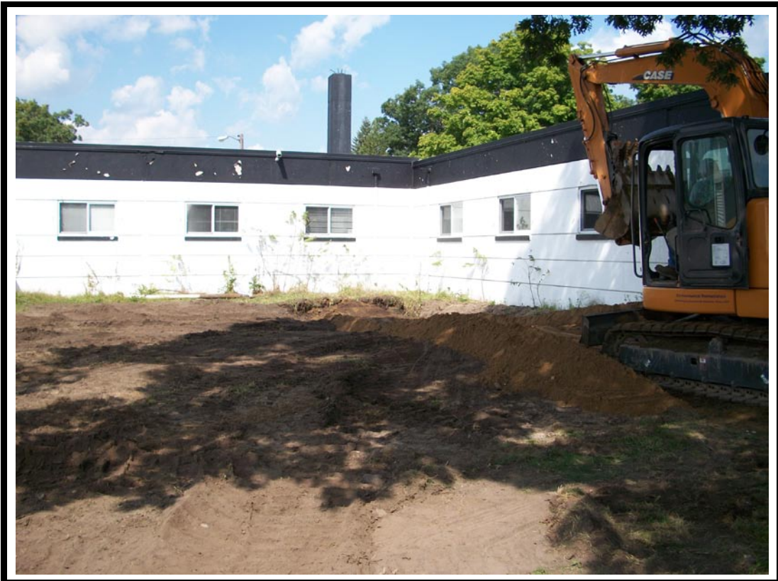
Photo No. 8: View of grading and leveling of tank pit after excavation.
