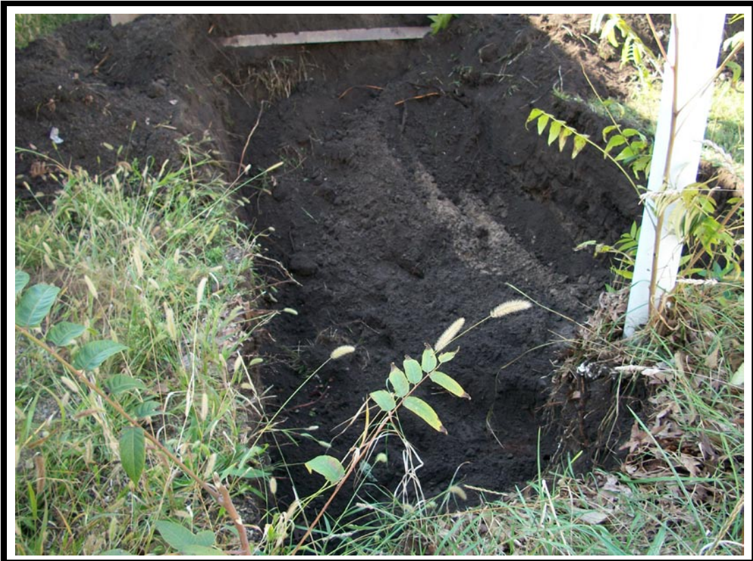
Photo No. 2: View looking south at excavated tank pit and top of the UST.
