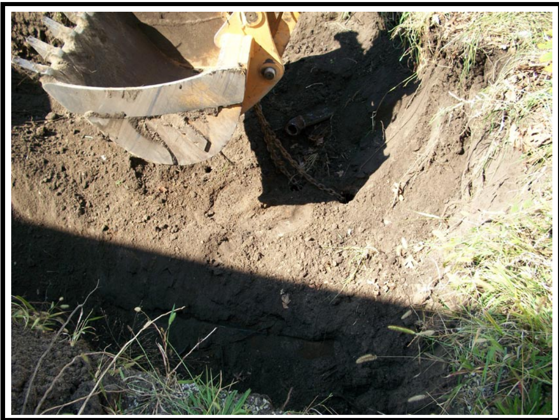
Photo No. 3: View looking west at northern end of exposed UST and broken off vent pipe connection.
