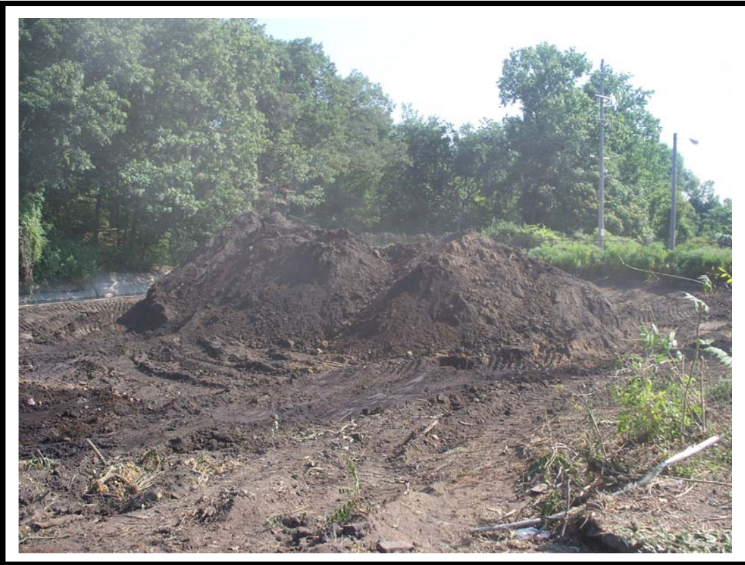
Photo No. 5: General view looking east of piled soils staged for removal during excavation.
