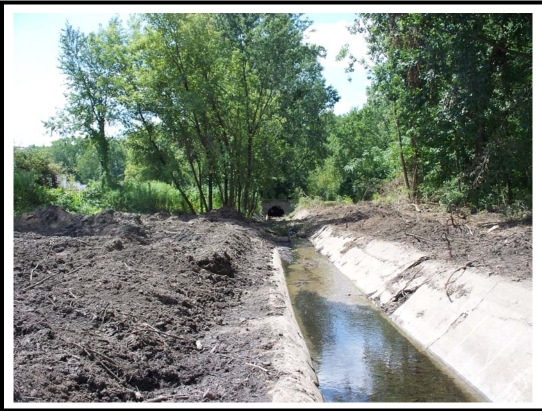
Photo No. 3: View looking west of Bowman Creek after clearing and grubbing of channel.
