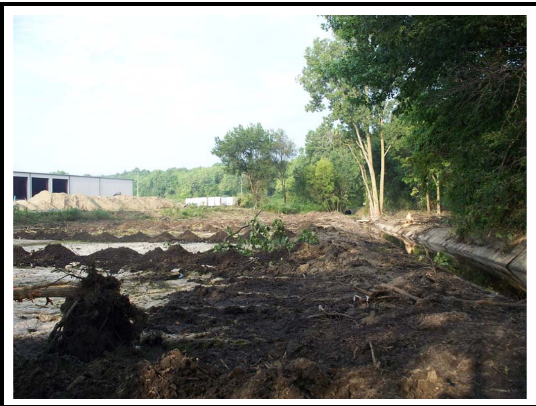
Photo No. 2: Further view of retention pond looking west prior to onset of remedial excavation.
