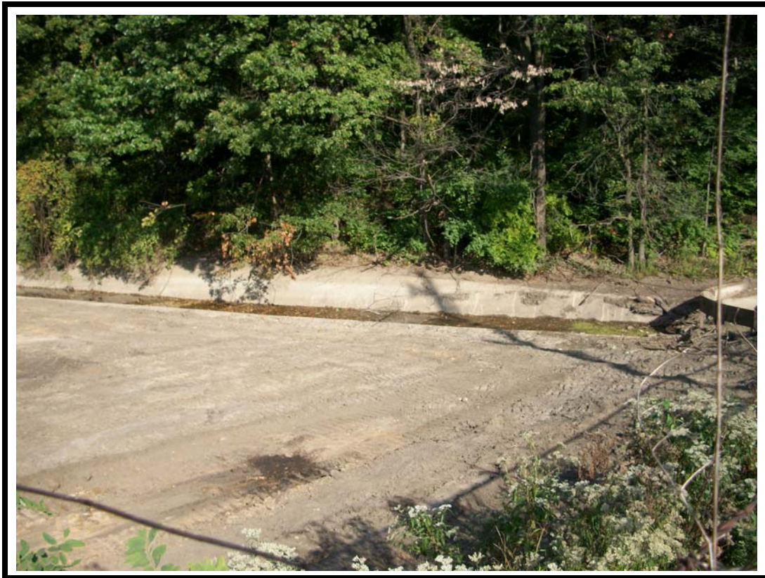
Photo No. 10: View of pond surface area looking south along eastern border after completion of excavation.
