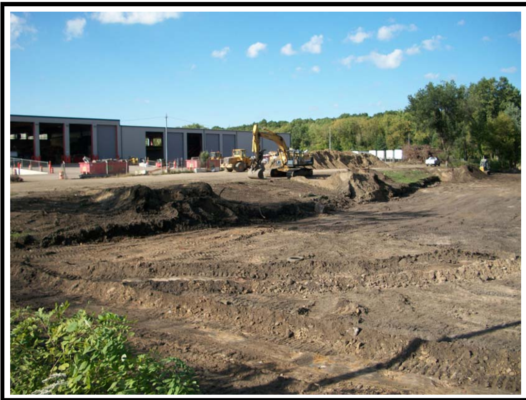
Photo No. 11: View looking northwest of graded pond surface area. Note piles of soils consisted of imported clean dirt used for ramp access.
