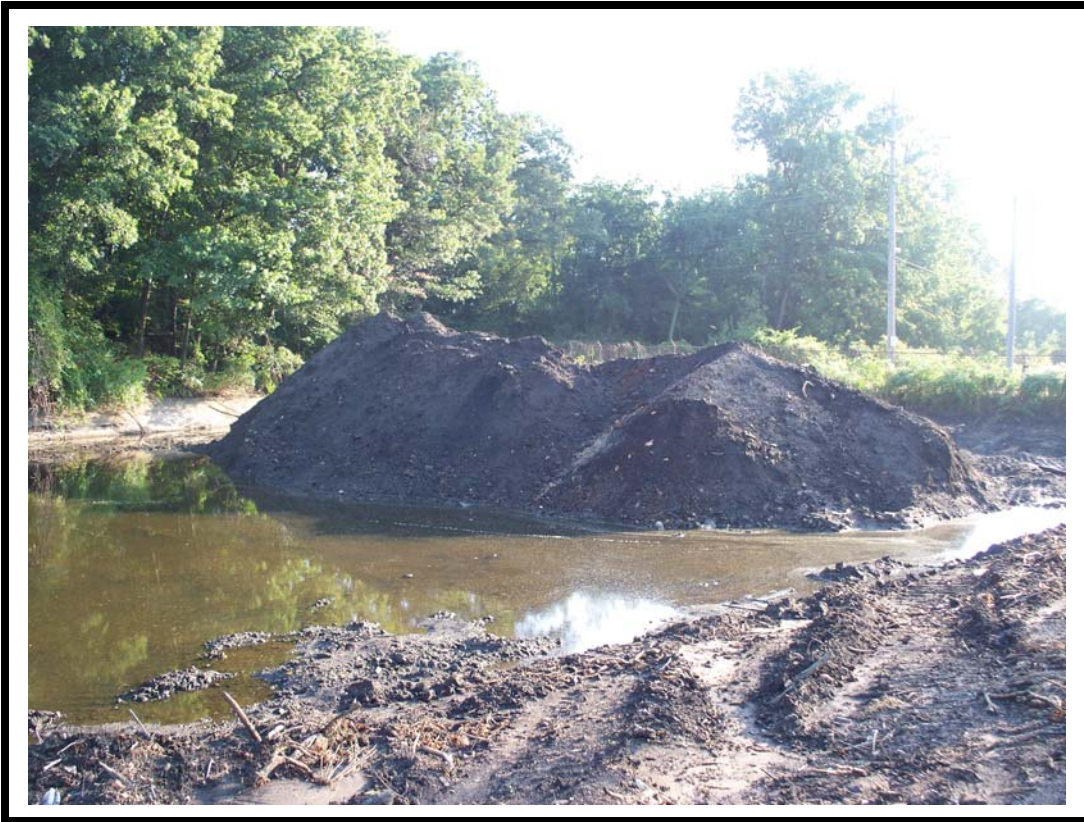
Photo No. 7: Additional view of ponded water after rainfall looking southeast.
