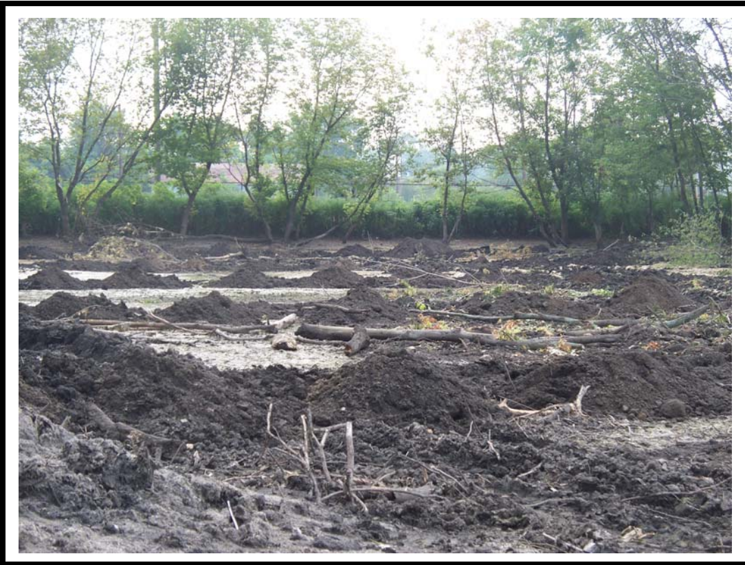
Photo No. 1: Overview looking east of retention pond surface area after drying and devegetation activities completed.
