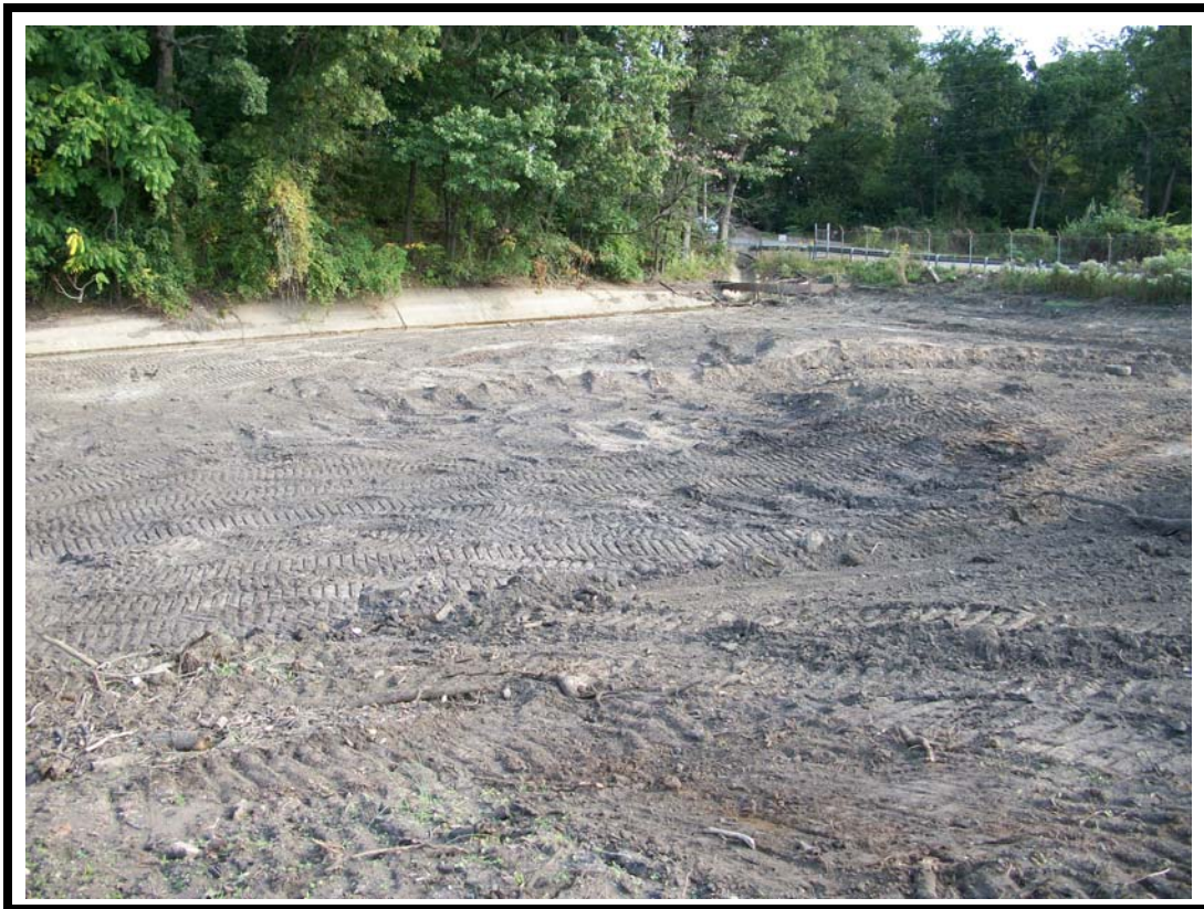
Photo No. 12: Close up view looking east of graded pond surface area of excavation completion.
