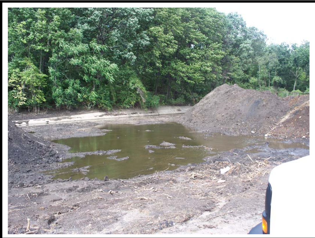
Photo No. 6: General view looking south of ponded rain water accumulated during course of excavation. Rainfall caused extensive delay in the completion of the project.
