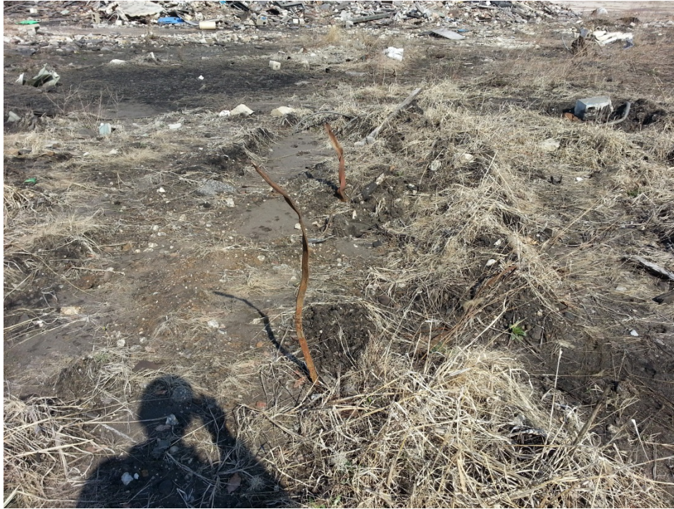
#3: Twisted rebar jutting out of foundry sand. This suggests there is more demolition debris buried beneath the sand.
