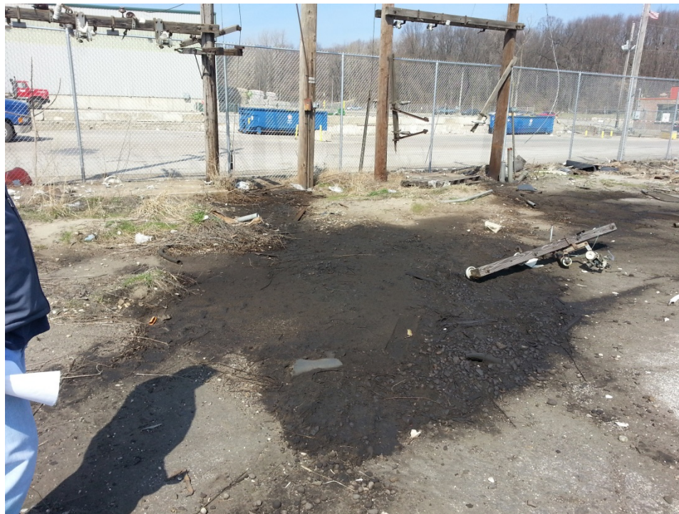
#28: As shown in this photo, the oily stain is sizeable and appears to flow out from a spot between two old utility poles.
