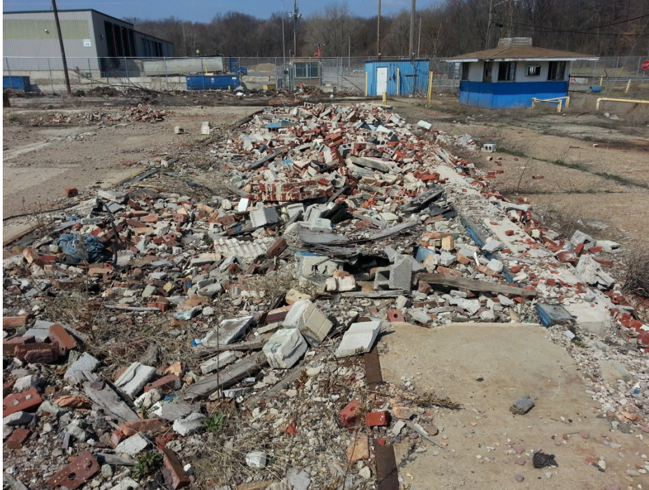
#35: This depression at the north of the former foundry building is full of demolition debris.
