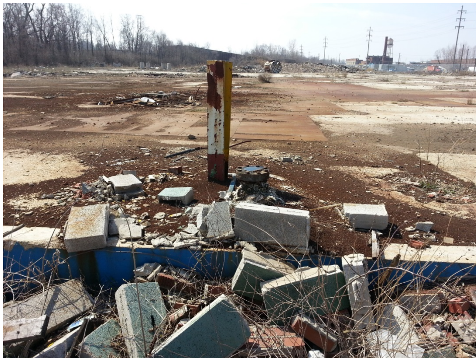
#36: This photo shows the other pipe at the northern edge of the former foundry building.
