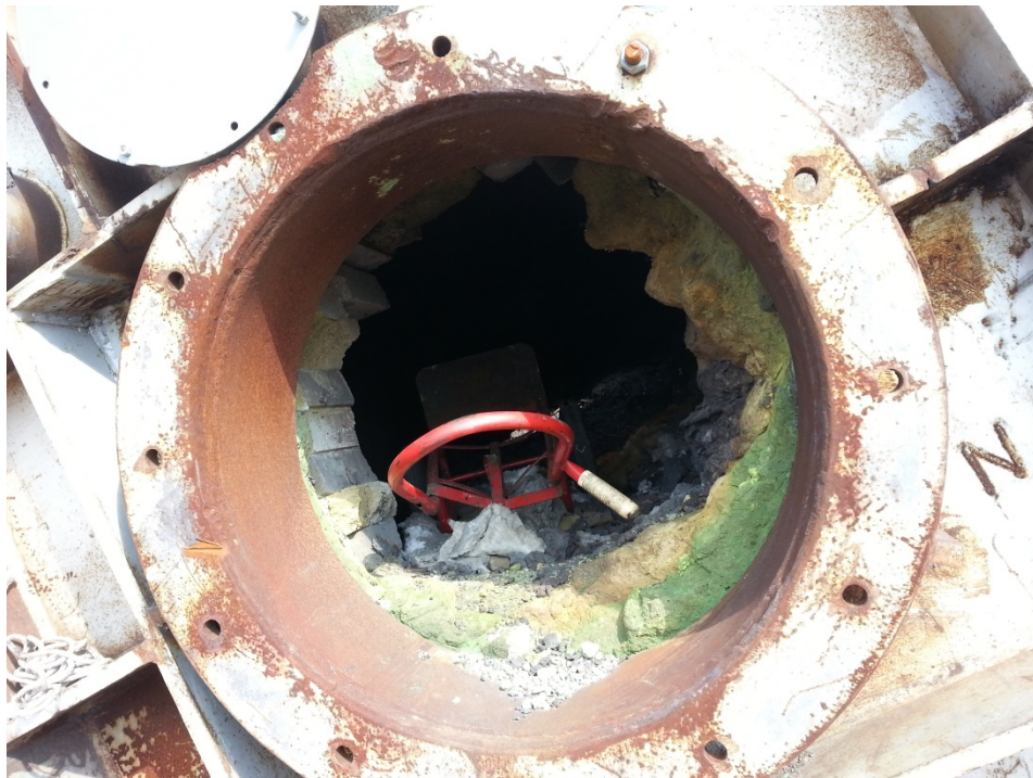
#22: The red object is a metal cargo dolly/hand cart. It is unclear who placed it there. The left side of the porthole appears to be refractory brick, while the right side appears to be coated with solidified slag.
