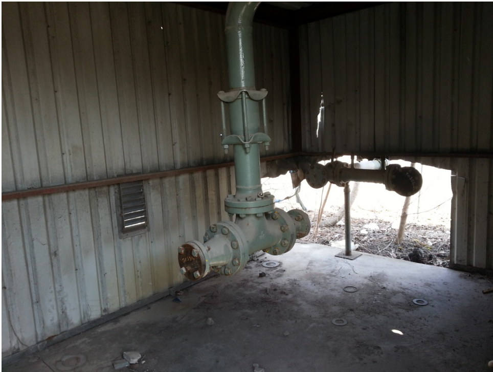
#32: Interior of the dilapidated gas house.
