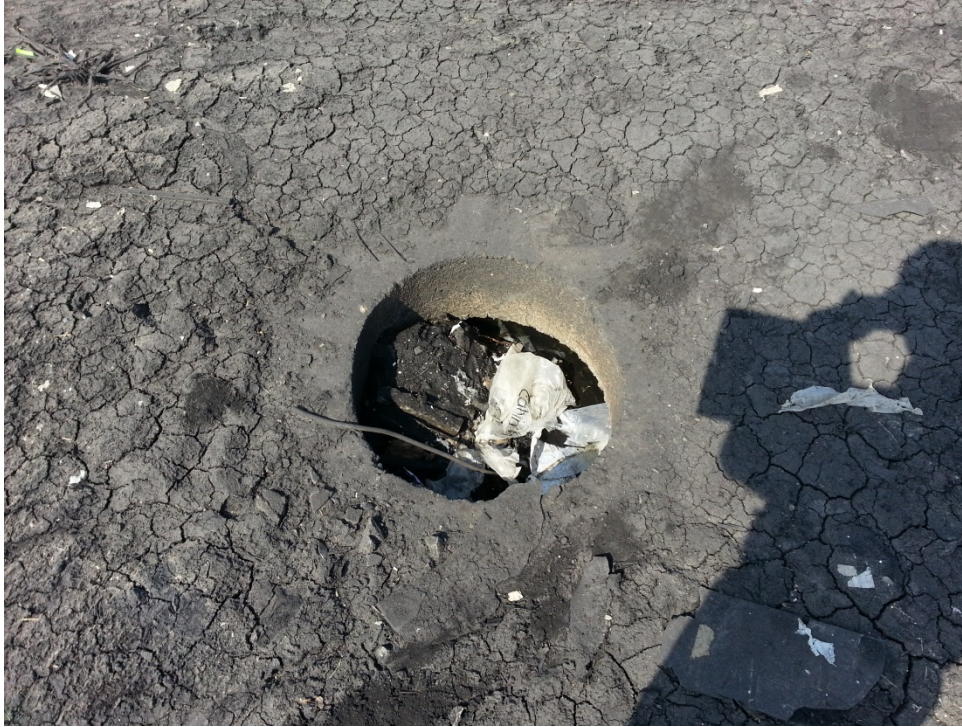
#17: One of the uncovered manholes, filled with garbage and water.
