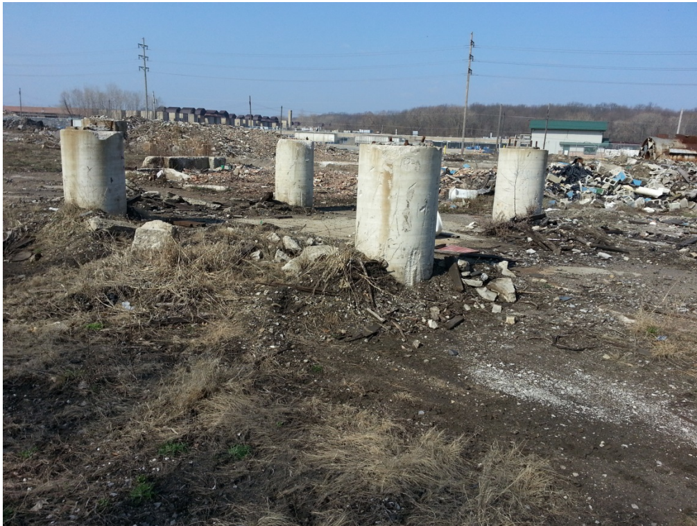
#2: Four large pillars at the eastern edge of the Property with debris piles in the background.
