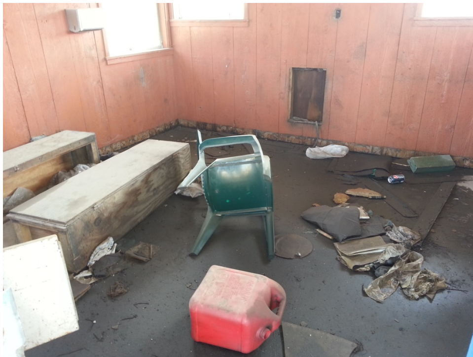
#34: Interior of the gate house. Two electrical fuses can be seen in this picture. The floor was entirely stained with a black oily substance similar to elsewhere on the Property. The only non-stained spot can be seen at the far right of the picture.
