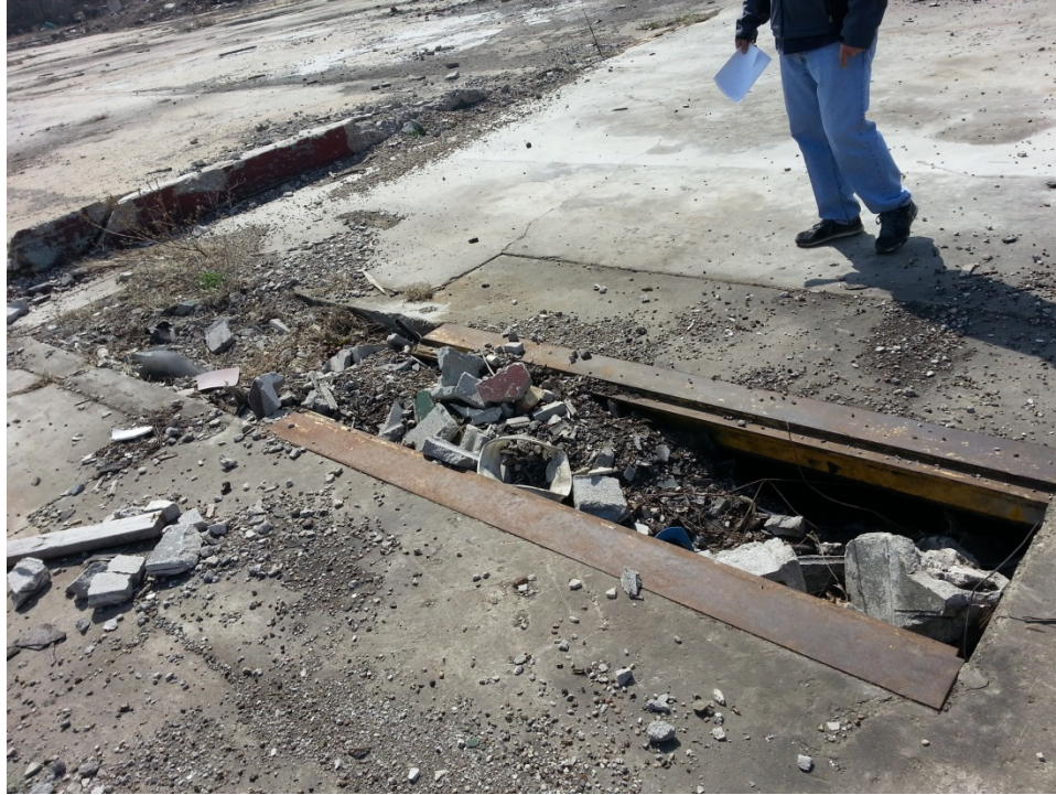
#29: One of several debris-filled pits found throughout the floor of the former foundry building.
