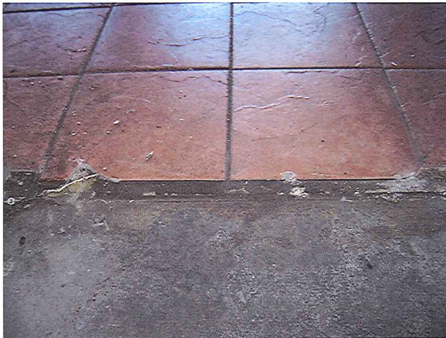
Brown floor tile (under red floor tile) and mastic (ACM) in entryway
