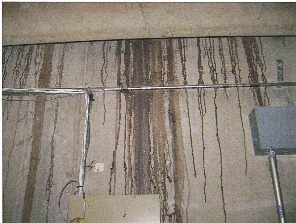
Staining on basement wall
