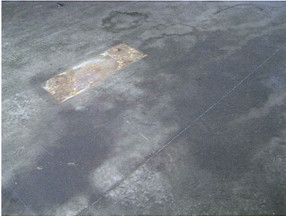
Staining on garage floor
