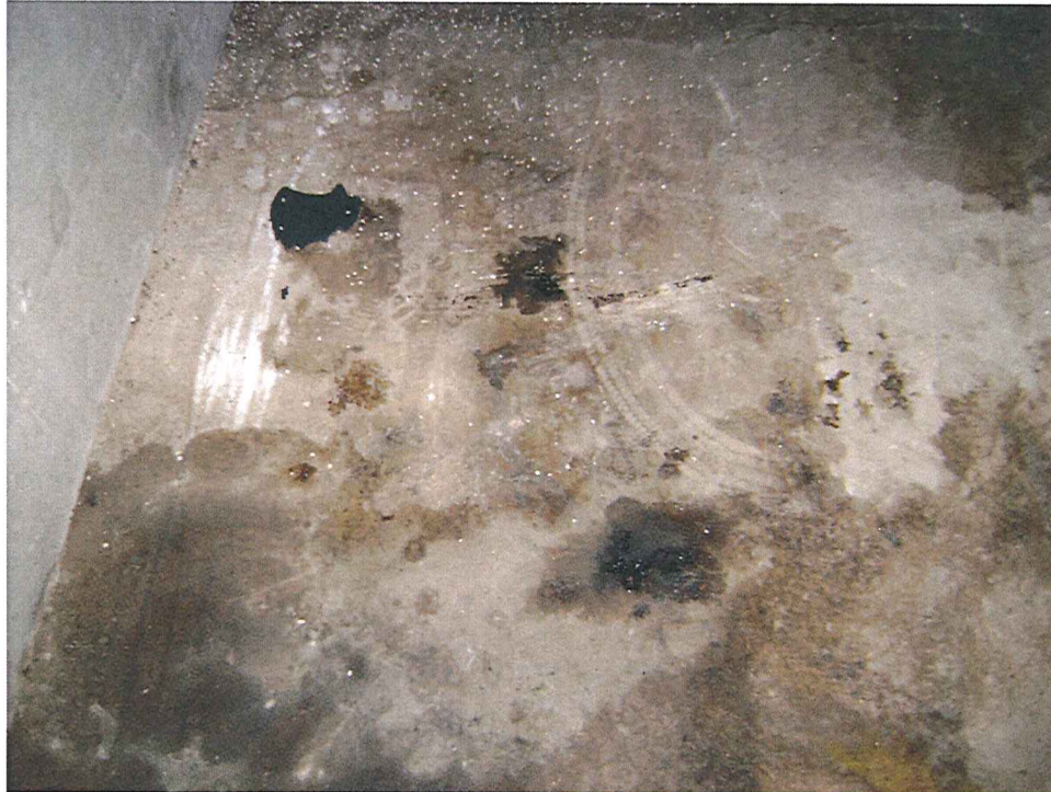
Staining on basement floor
