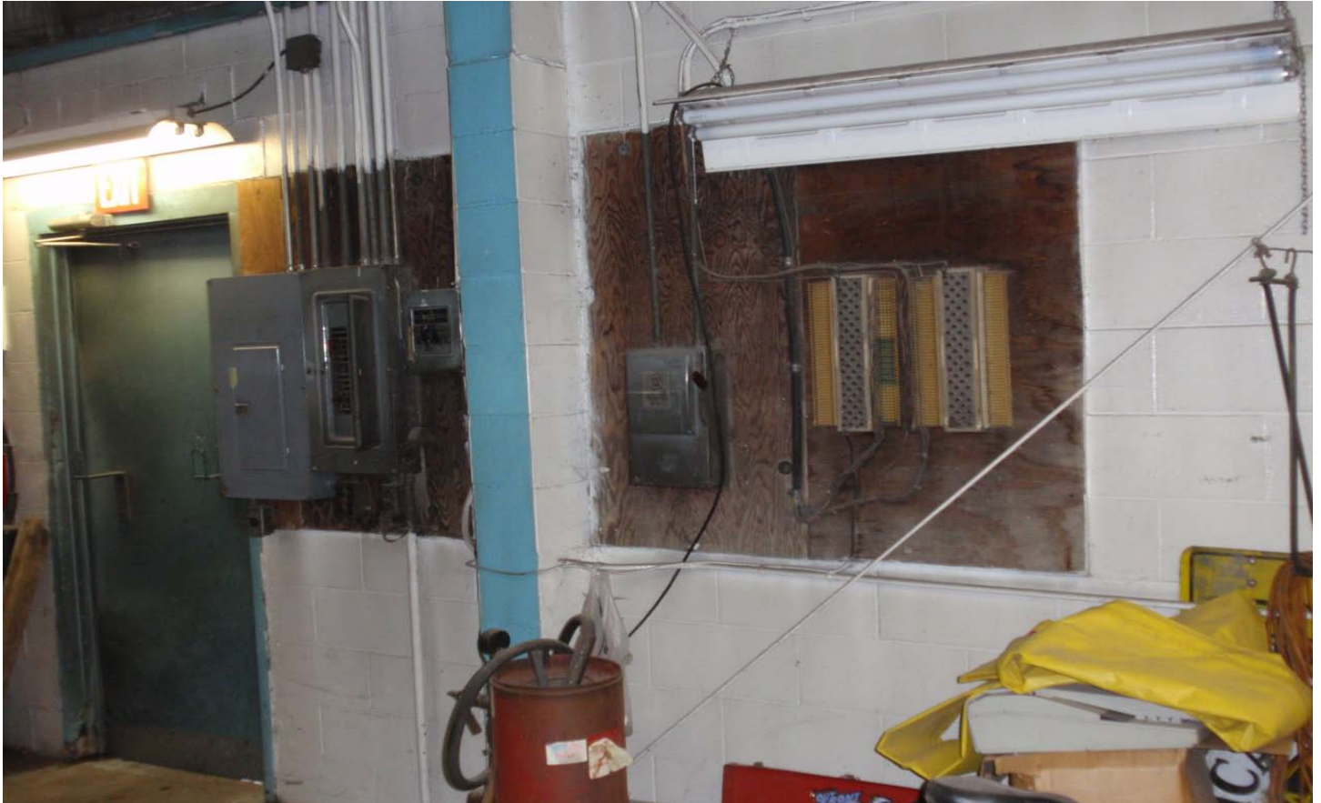
Electrical Switch Boards in Main Structure
