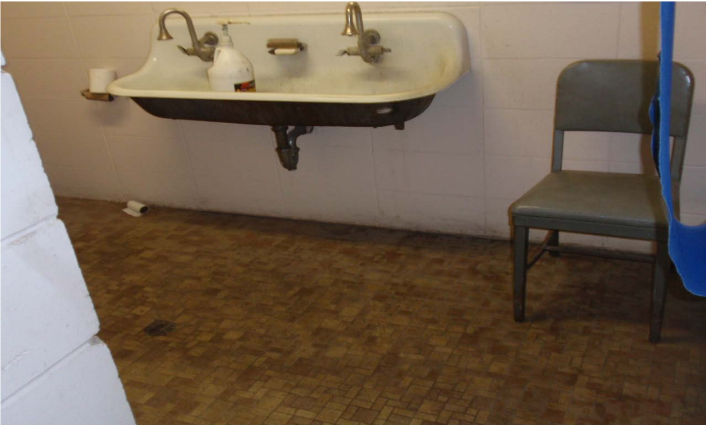
Bathroom Floor Drain
