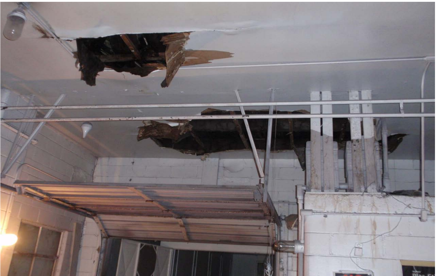
Water Damage in Paint Shop Structure
