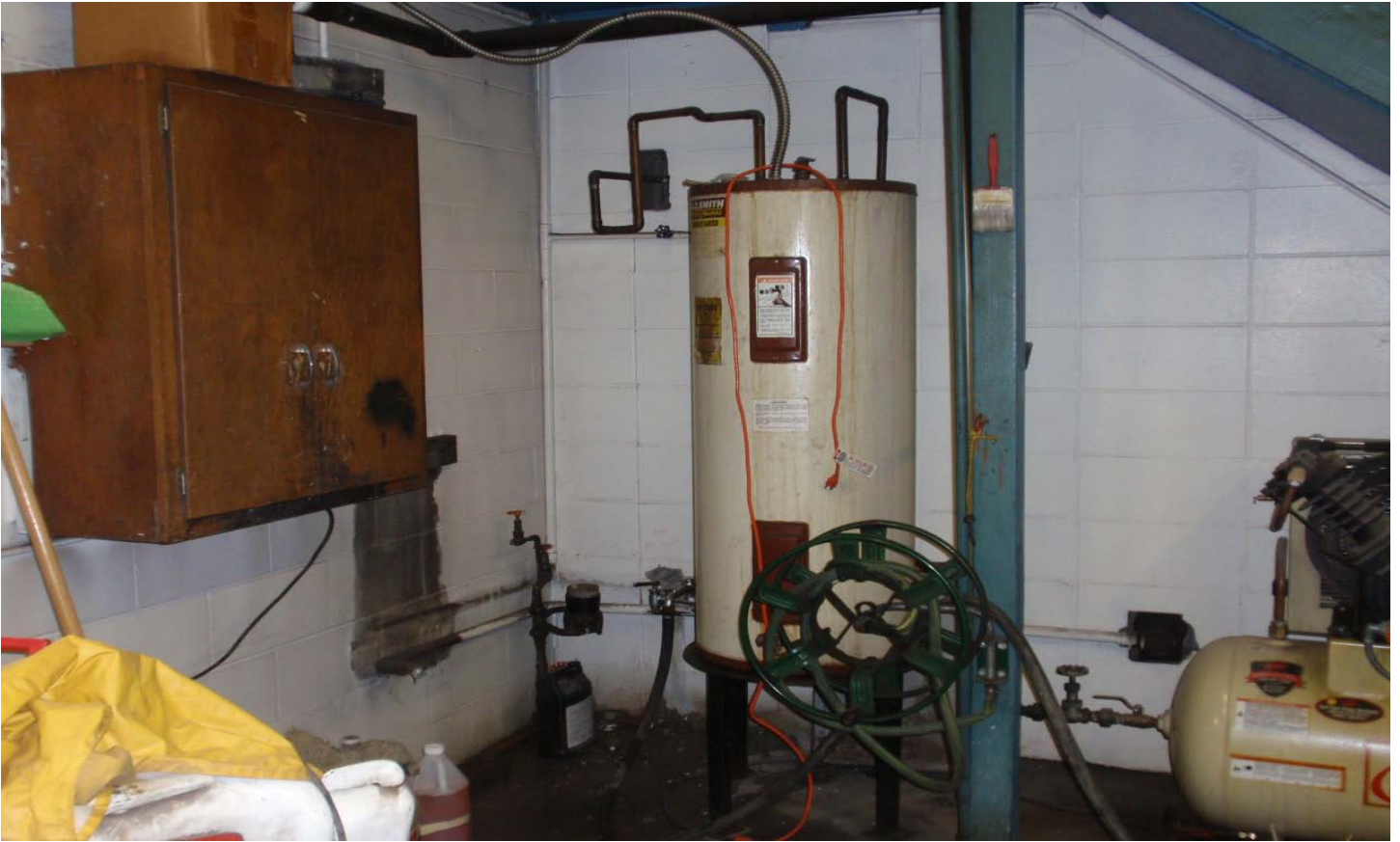
Water Heater in Main Structure
