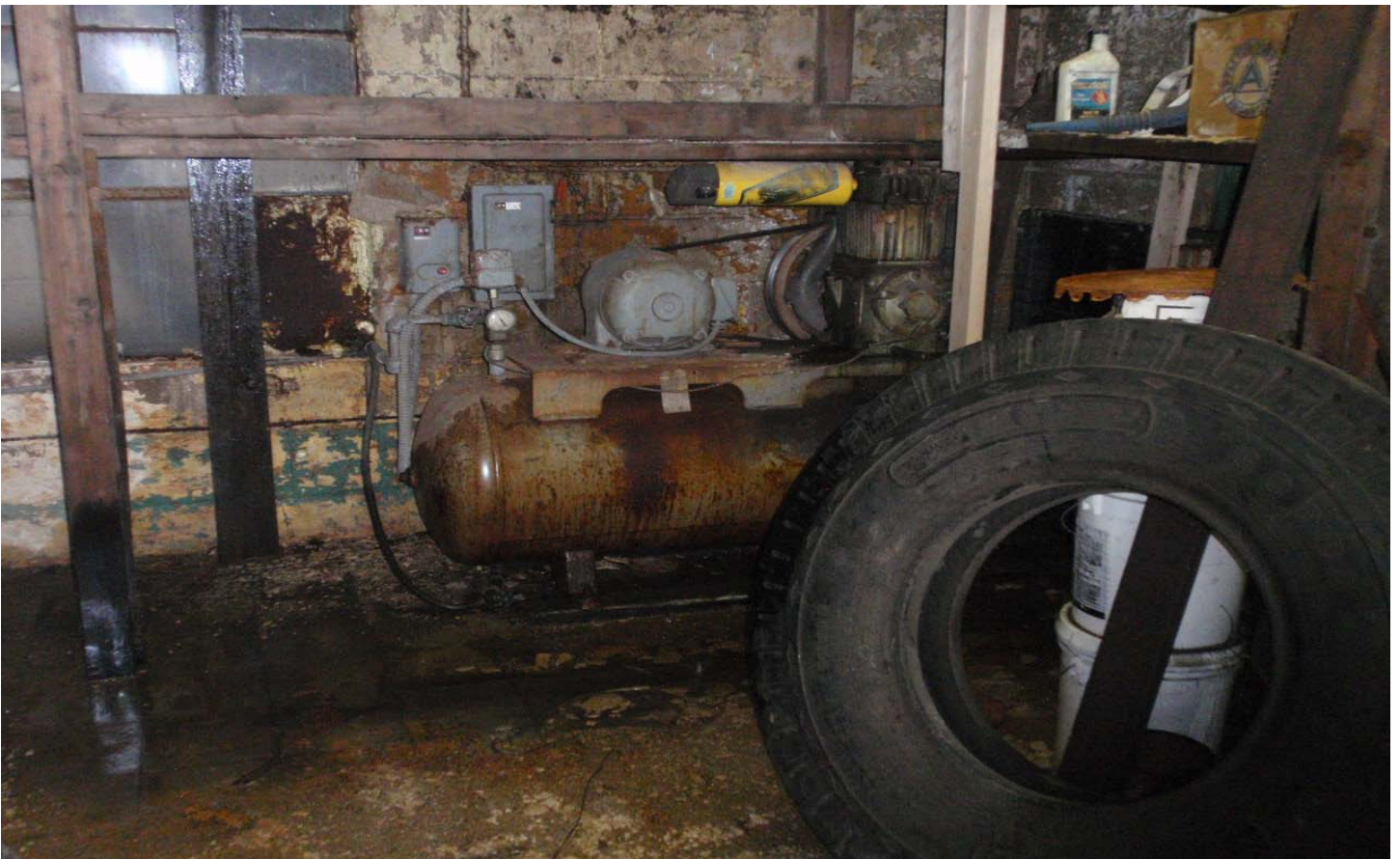
Air Compressor inside Storage Structure
