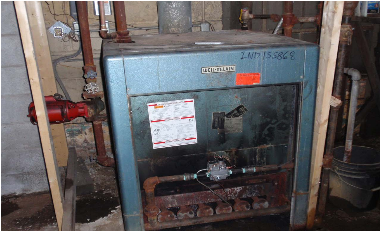
Boiler in Storage Structure
