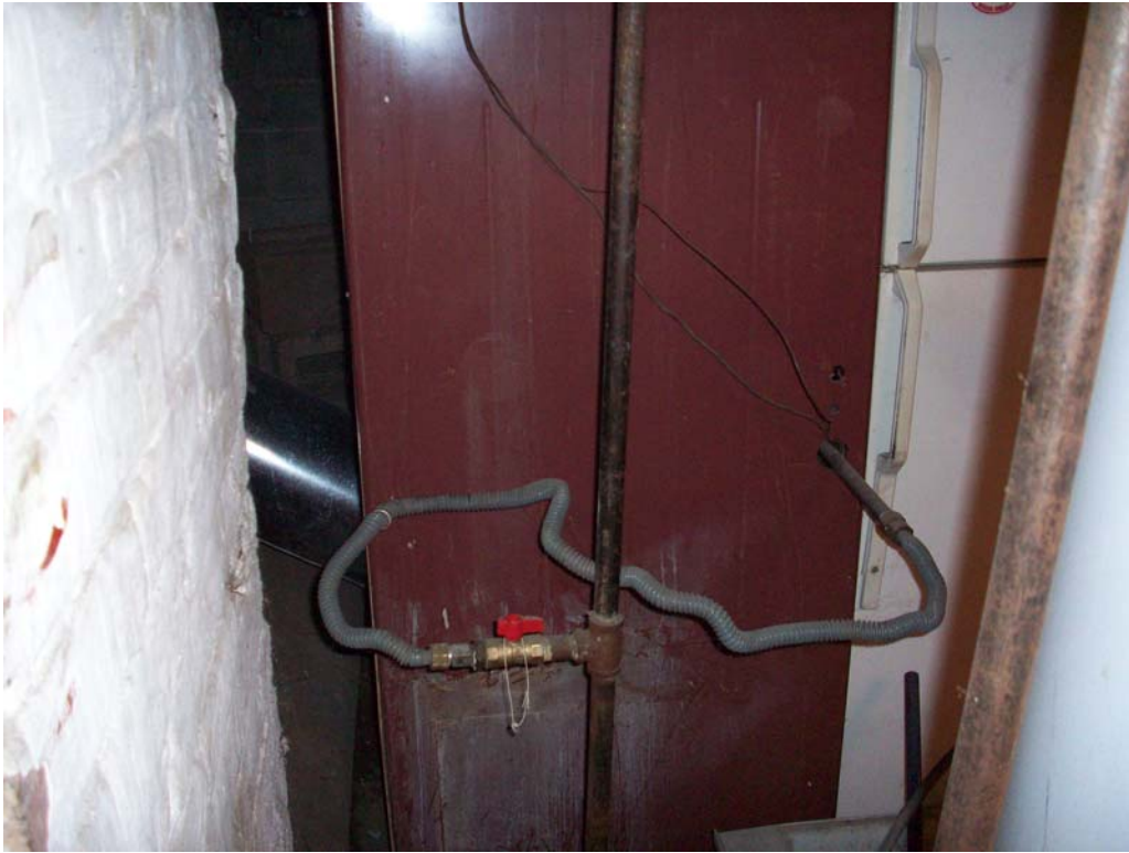
Basement (gas connection for forced-air furnace)
