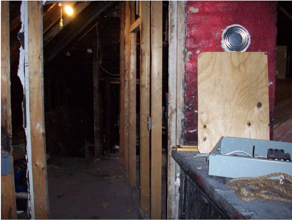
Second (upper) level, fire damage
