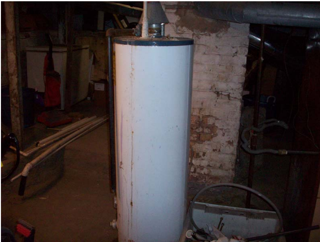
Basement (water heater, natural gas)
