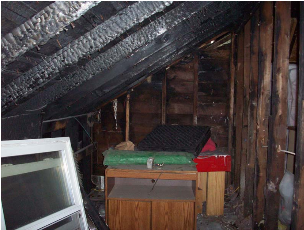
Second (upper) level, fire damage
