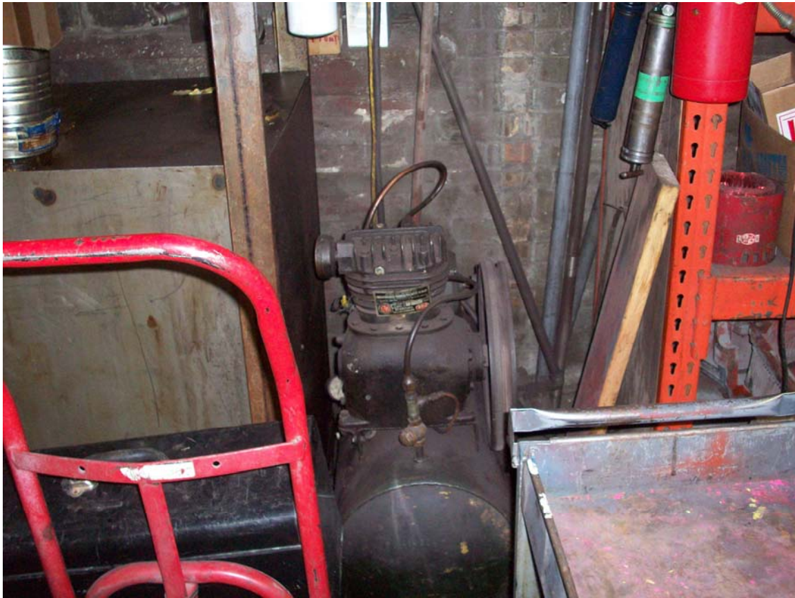
Air compressor unit adjacent to waste oil furnace (atomizer)
