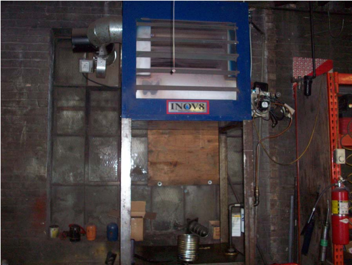
Ceiling mounted gas heaters for workshop
