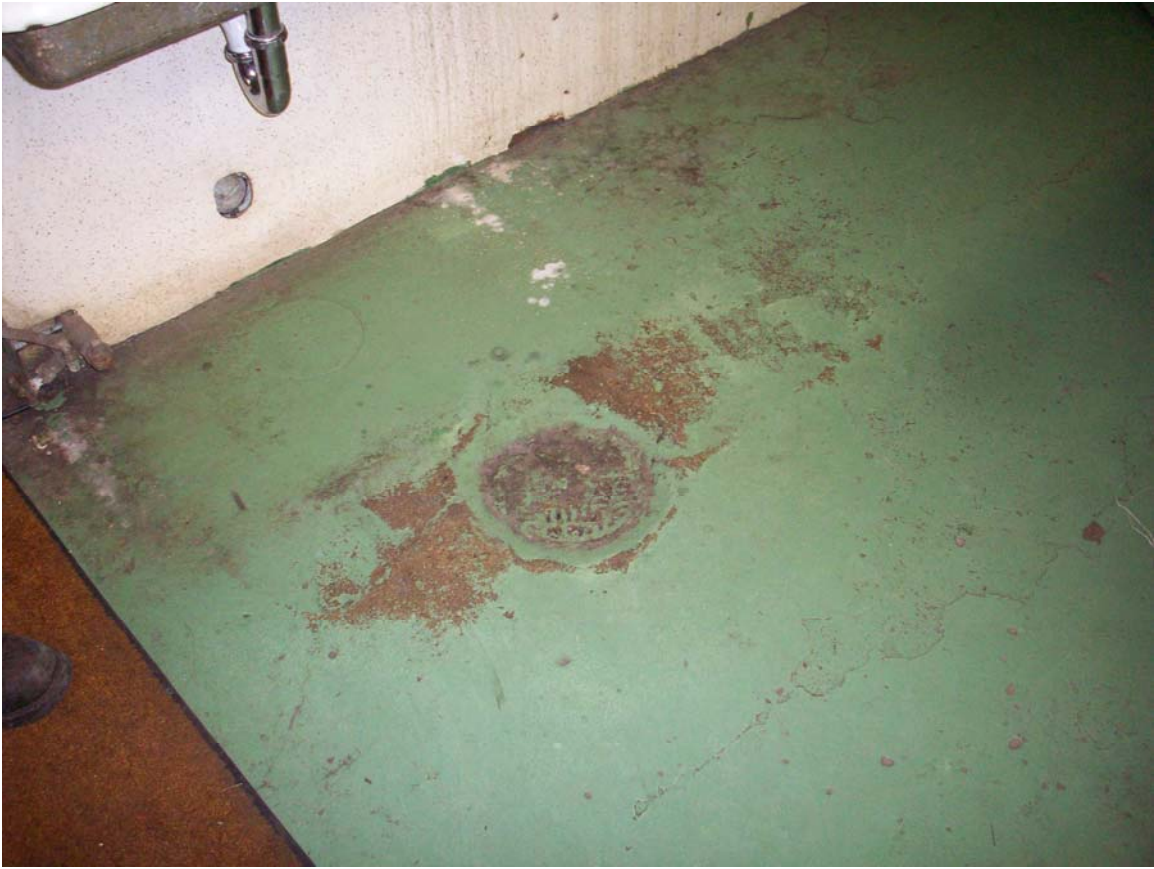
Floor drain (one of several) in shop area
