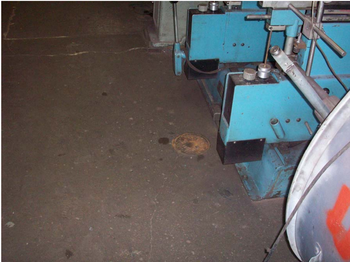
Floor drain in workshop area
