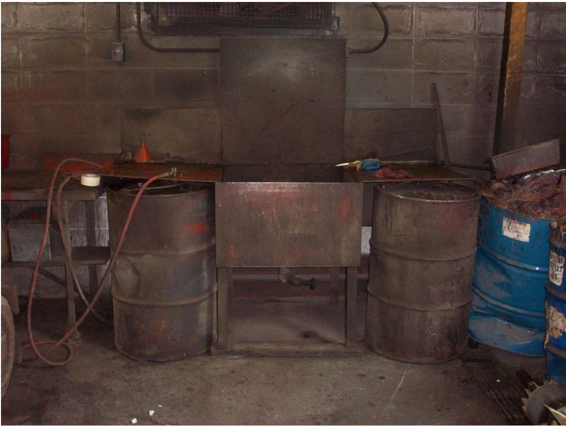
Degreaser – note adjacent floor drain
