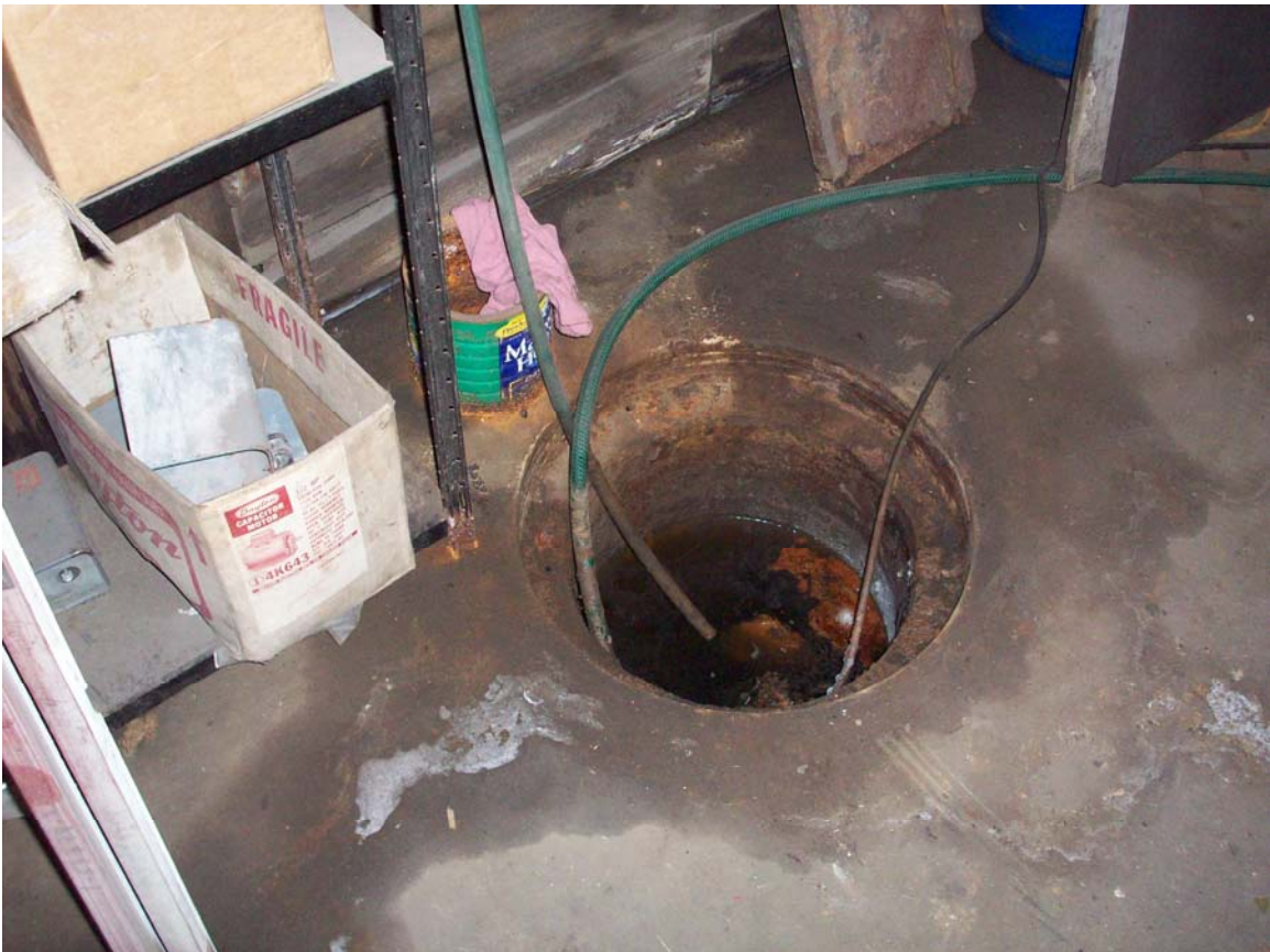
Sump – reportedly not in use (note staining of area)
