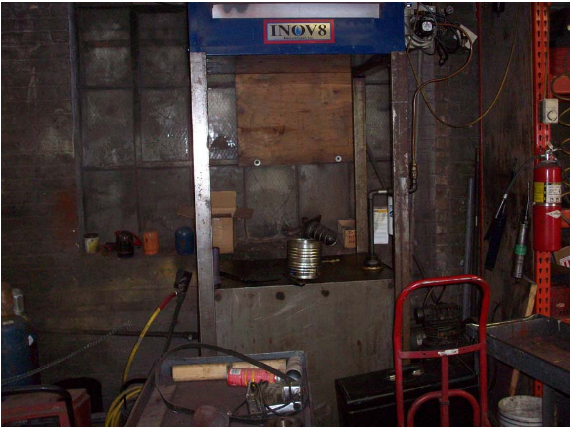
Furnace for waste oil
