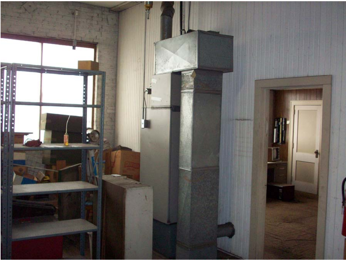
One of three gas forced air furnaces (upstairs)
