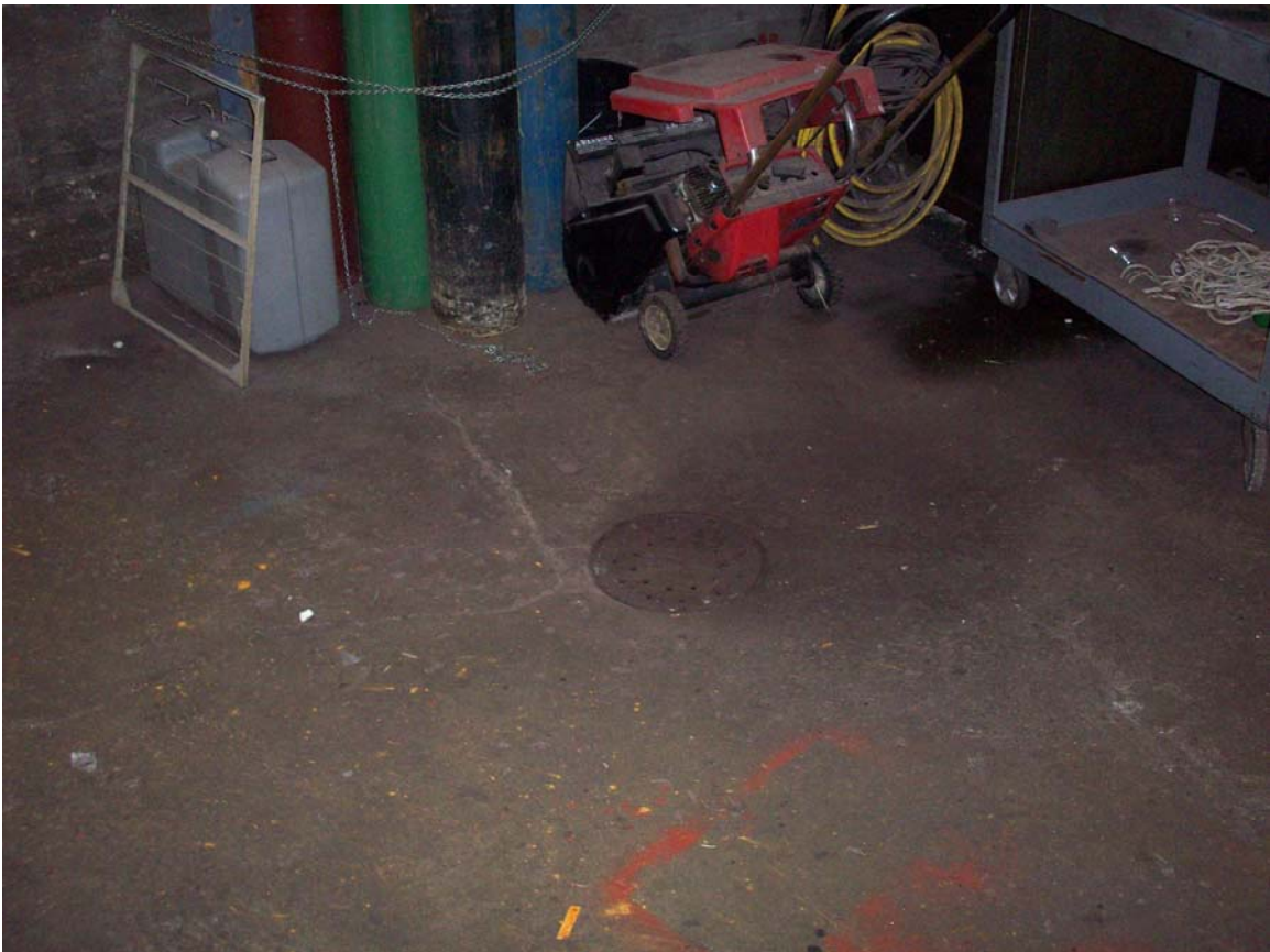
Floor drain in shop area – note staining of floors
