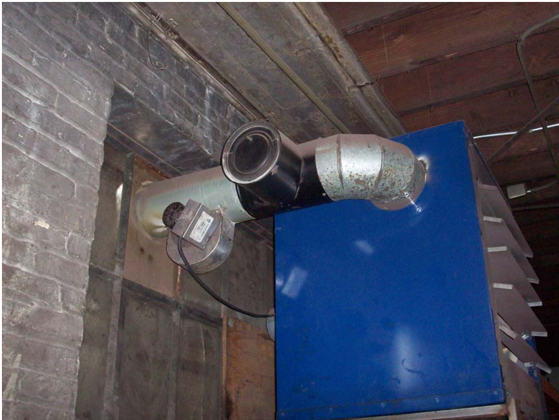
Point of emissions discharge from waste oil furnace
