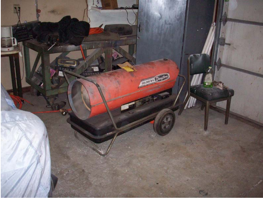
Kerosene heater (natural gas service terminated)
