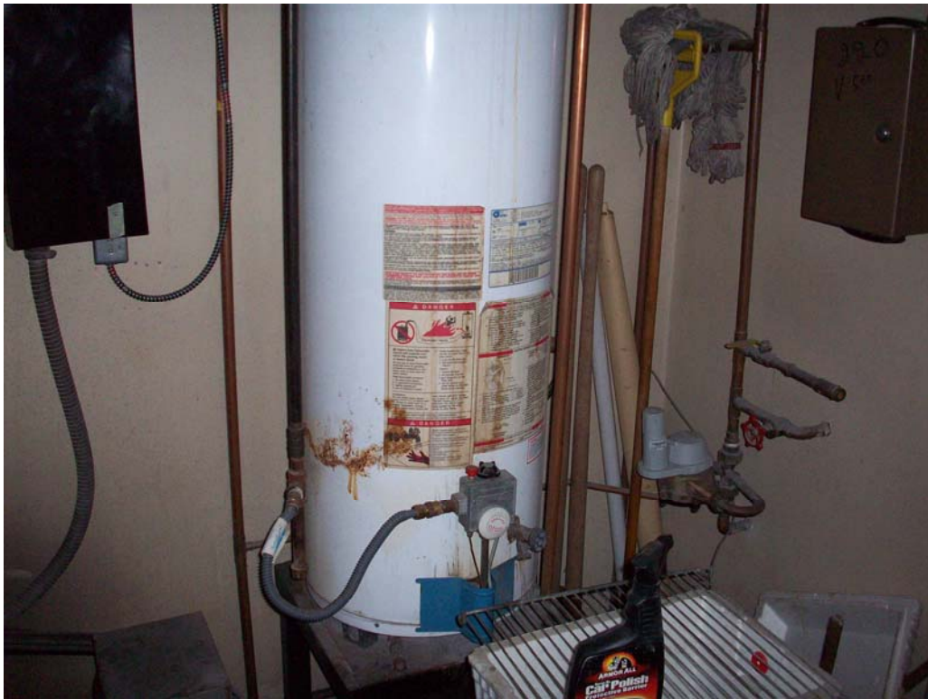
Water heater – non functioning (natural gas service terminated)
