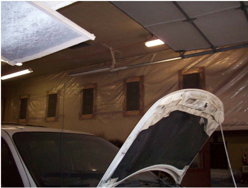
Western bay of garage, appearance of spray paint booth
