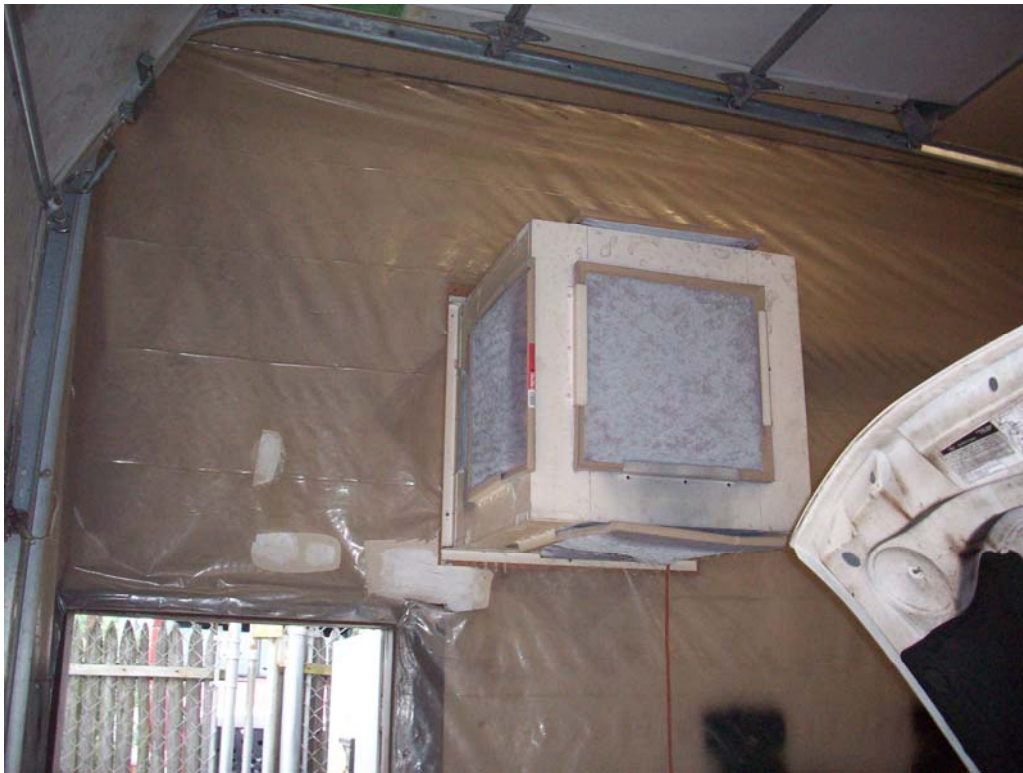
Air filtration systems of west bay
