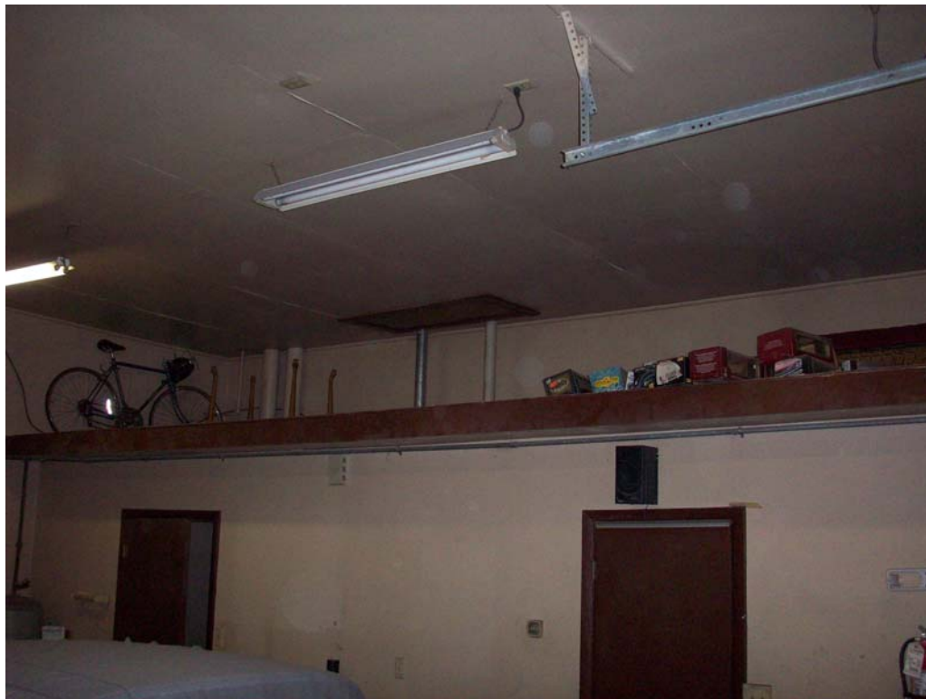
Gas furnace lines – located in attic area (non-functioning)
