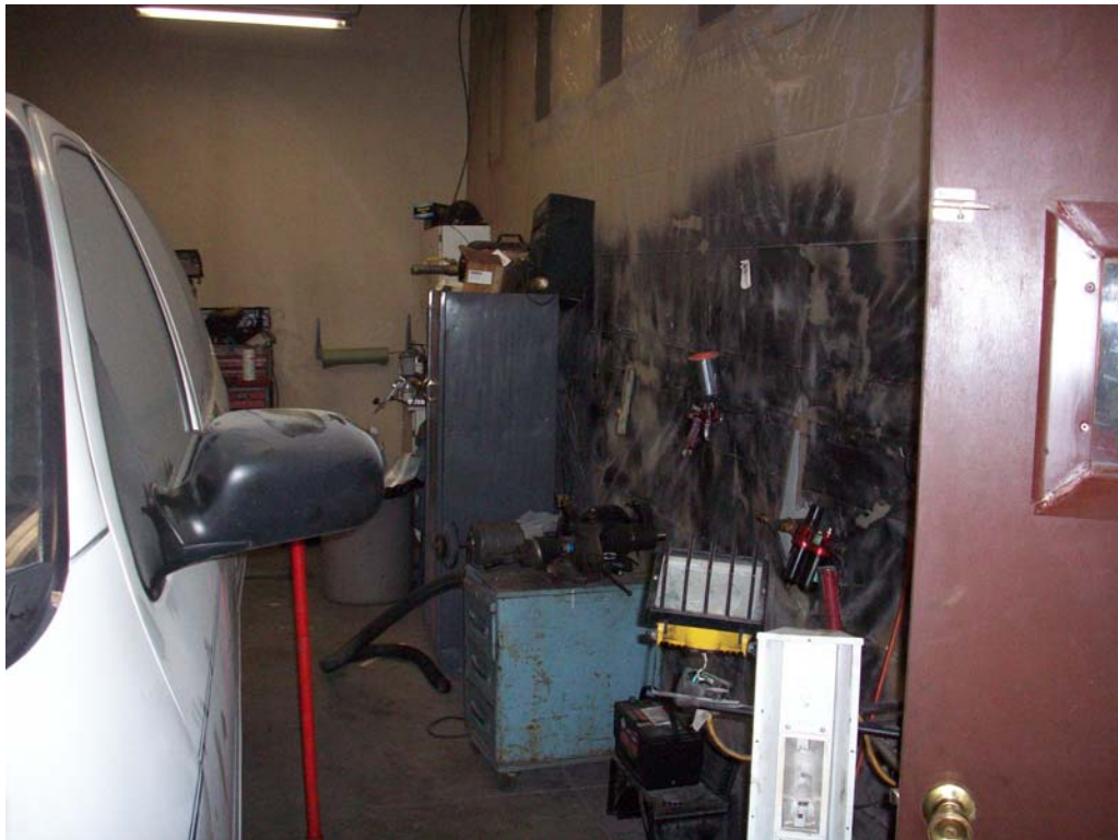
Indications of spray painting on wall of west bay
