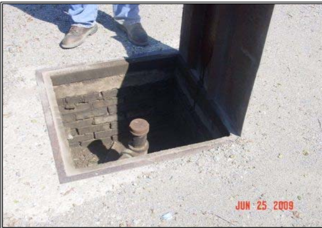
PHOTO 8: Square metal cover over the top of a fill port.
