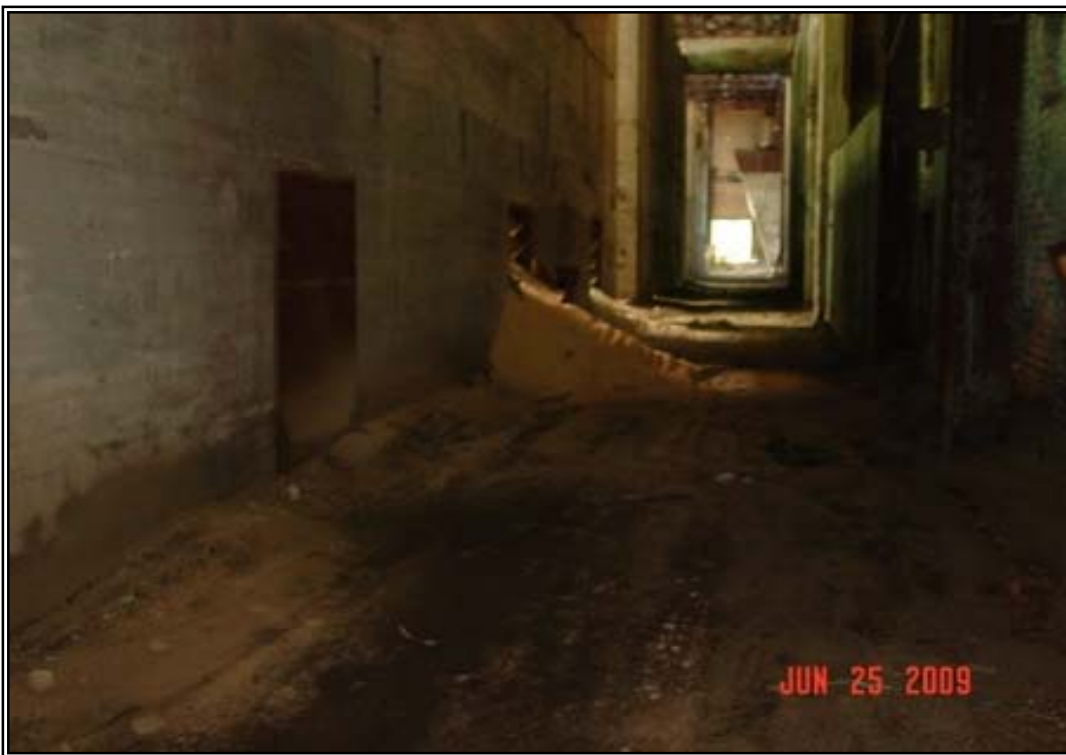
PHOTO 12: Corroded doors to coke pits have allowed sands to pour into corridor.
