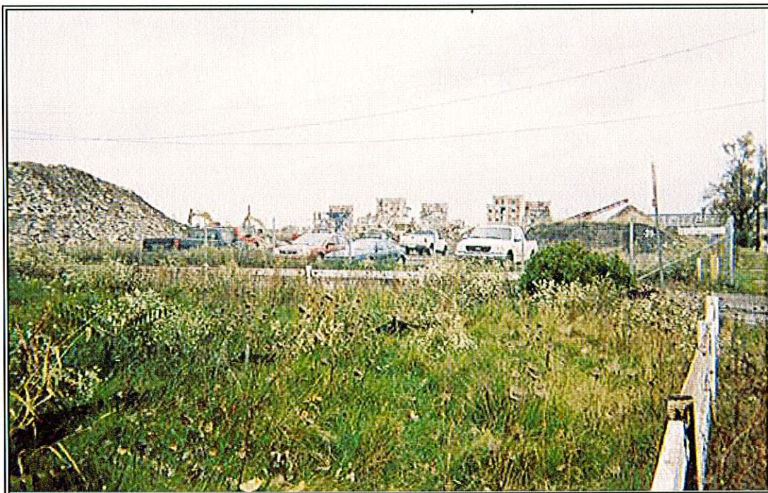
PHOTO 8: North-facing view of the former Allied Products Corporation property, currently undergoing demolition and redevelopment.
