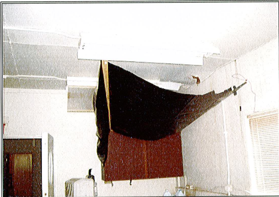
PHOTO 4: Tarp erected in a room of the main building where the roof leaks.
