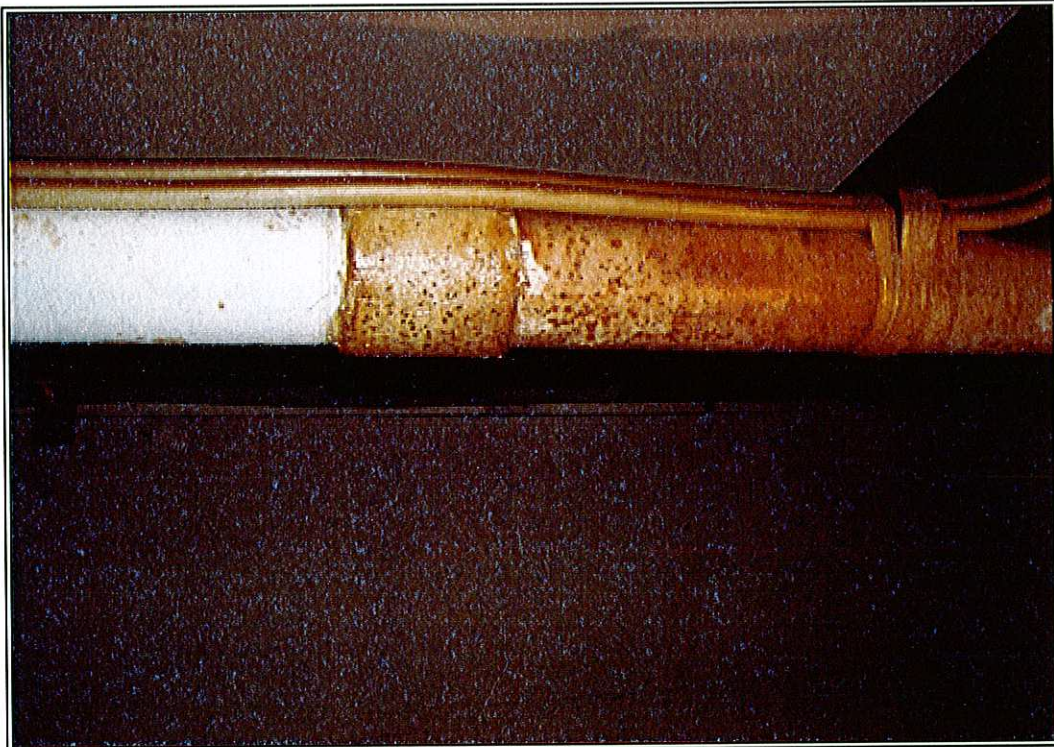
PHOTO 14: Junction in suspected UST pipe where it appears to be leaking. Film on pipe has a petroleum odor.
