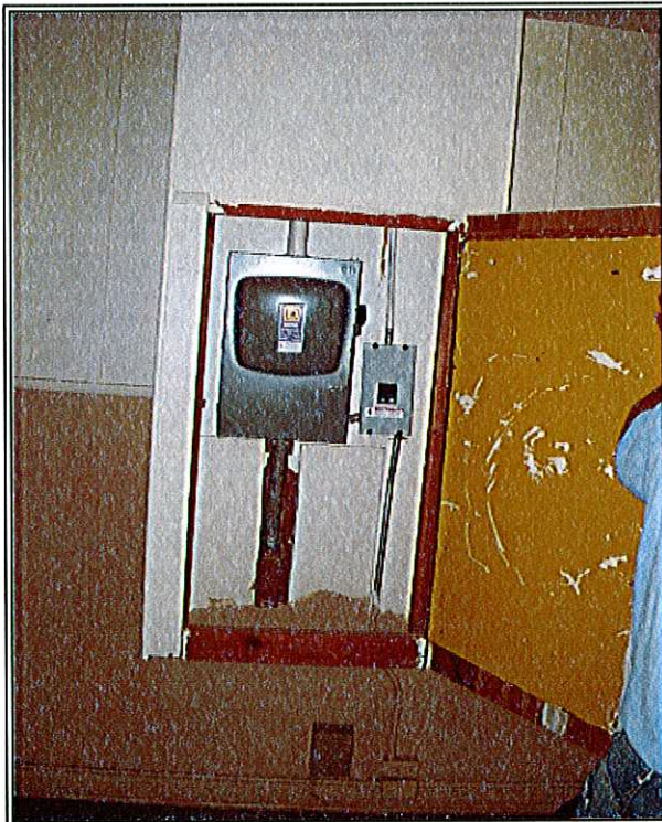
PHOTO 2: Power source in main room in the main building.
