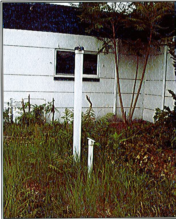
PHOTO 21: Suspected fill and vent pipes on the southern portion of the building.
