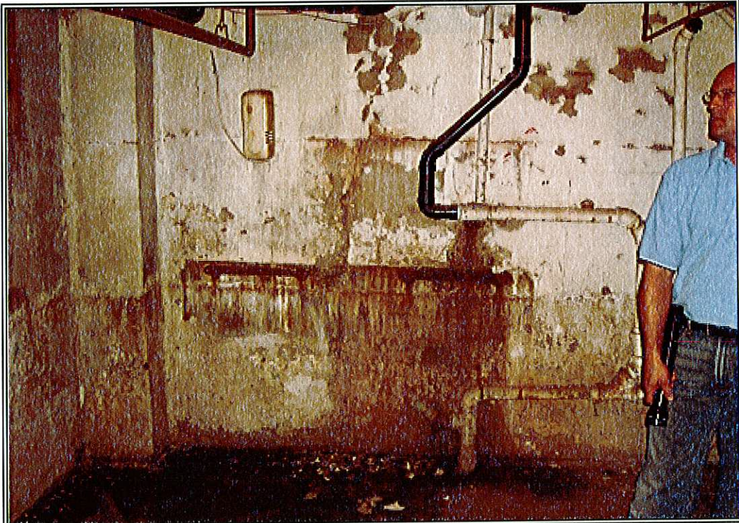
PHOTO 9: Staining on walls where water appears to seep in through the concrete.
