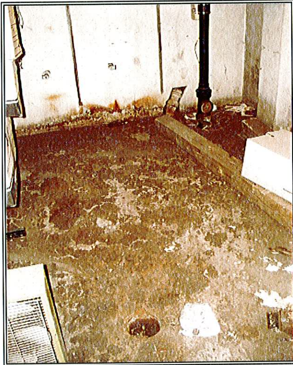
PHOTO 7: Drain in basement of the building.
