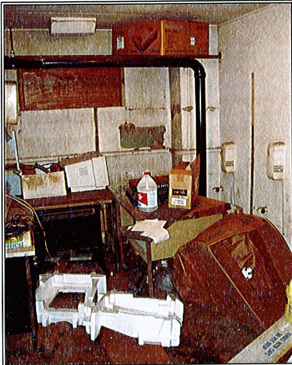
PHOTO 11: Stored supplies and debris were found throughout the ground floor and the basement.
