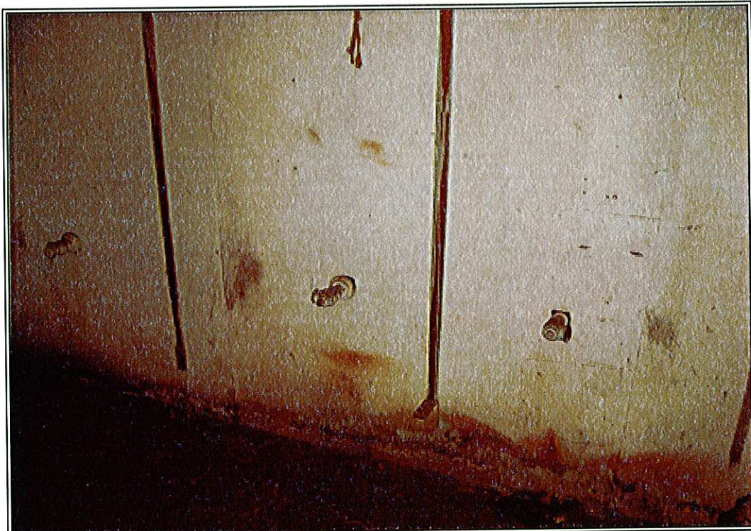
PHOTO 8: Walls exhibit staining from possible flooding.
