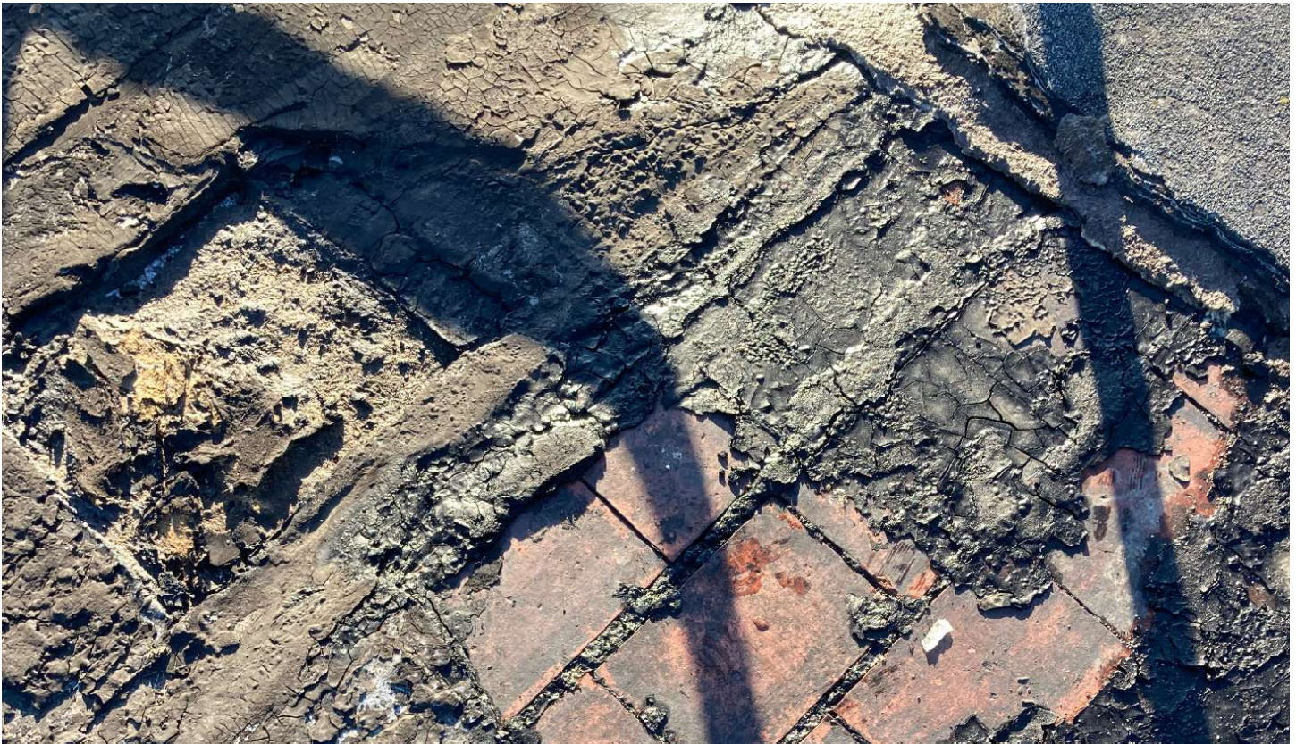
Photo 23 - Roof condition at top of Monitor Roof (bricks above concrete wall below)
