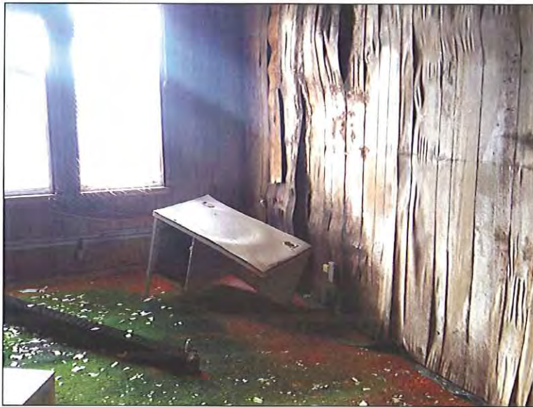
Third Floor - Southwest location - Moisture related staining/damage and visible microbial growth on various building materials and contents.
