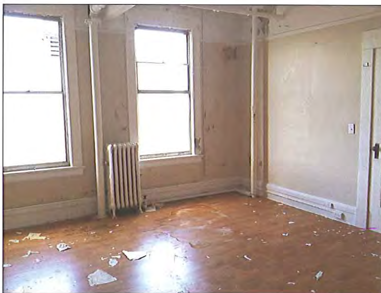
Fourth Floor - North location - Moisture related staining/damage on building materials
