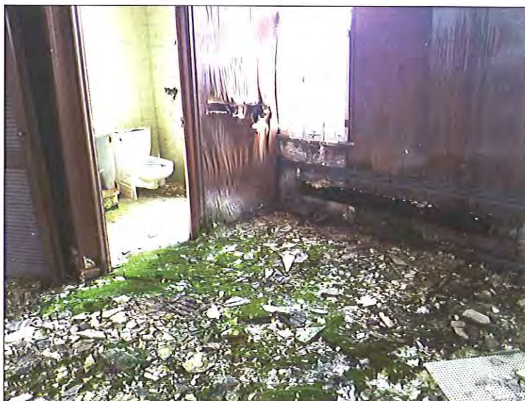
Fifth Floor - West location - Visible microbial growth as well as moisture related staining/damage on multiple building materials and contents
