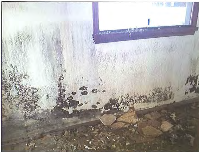
Fifth Floor - South location - Room 512 - Visible mold growth as well as moisture related staining/damage on multiple building materials.
