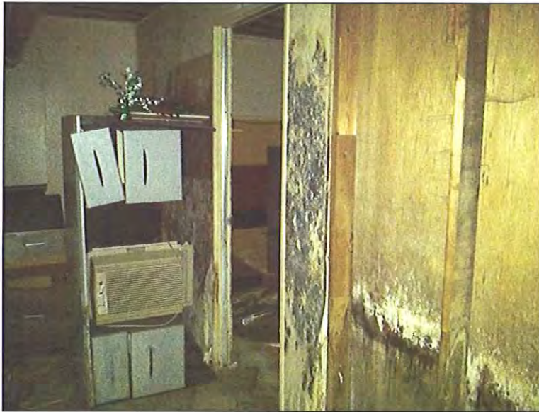
Basement - Center location - Visible mold growth on drywall and wooden building materials
