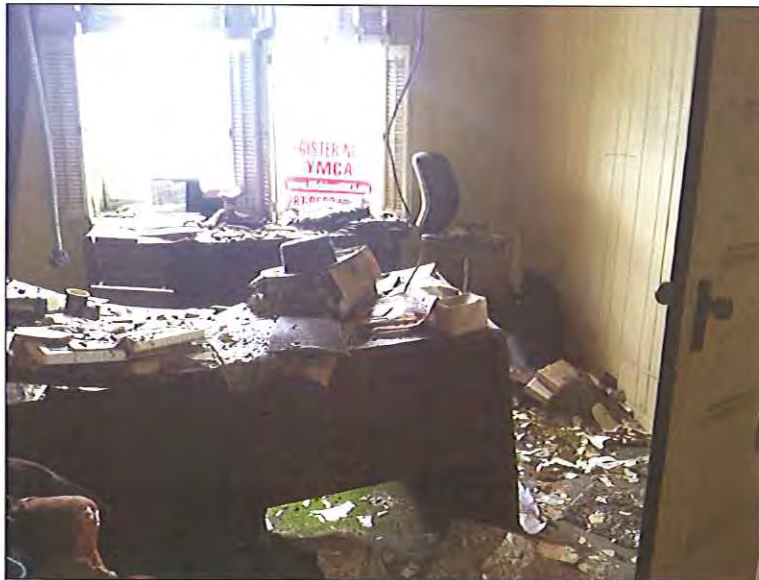
Second Floor - West location - Visible microbial growth and moisture related staining/damage present on multiple building materials and contents
