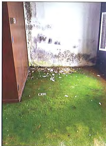
Fifth Floor - Northwest corner room - Visible microbial growth on the wall and carpet
