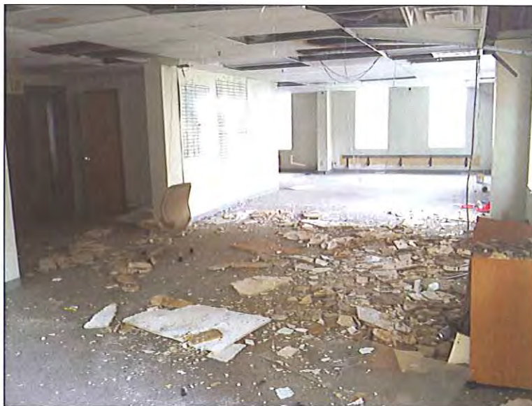
Third Floor - East location - Moisture staining/damaged ceiling tiles on the floor
