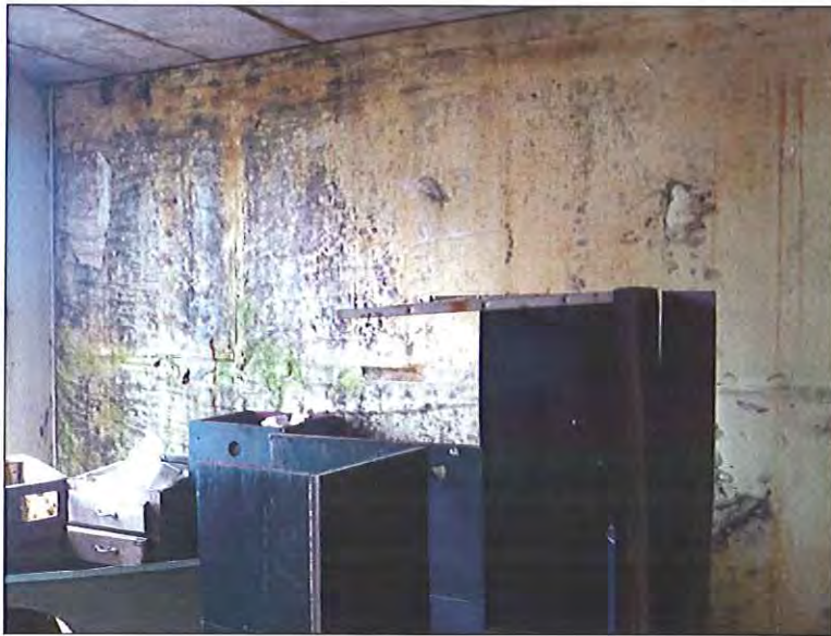
Second Floor - Southwest location - Visible microbial growth and moisture related staining/damage present on multiple building materials and contents
