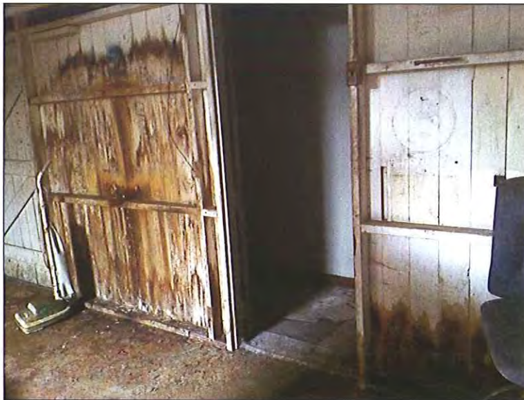
Basement - South location - Moisture related staining and mold growth on wooden wall paneling
