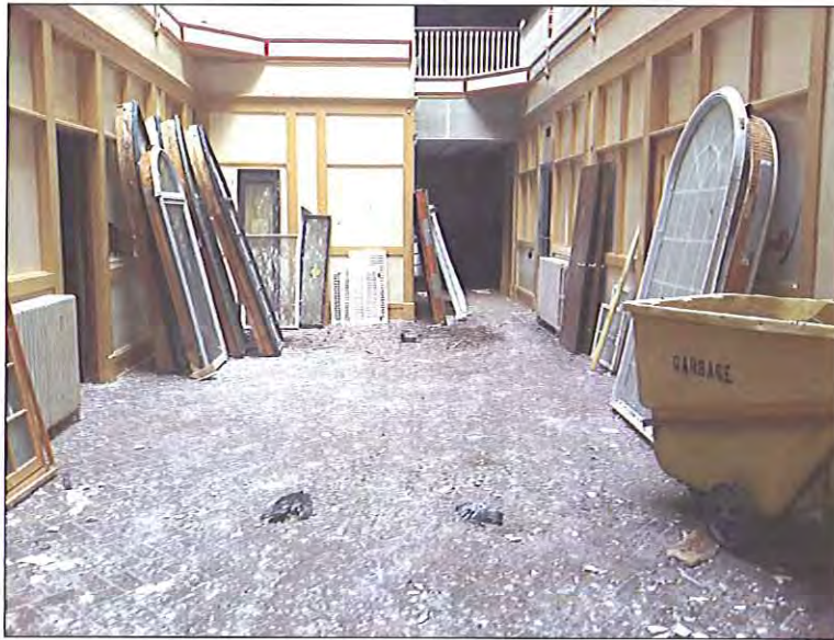
First Floor - Center location - Avian fecal matter present on surfaces throughout this area, in addition to multiple bird carcasses
