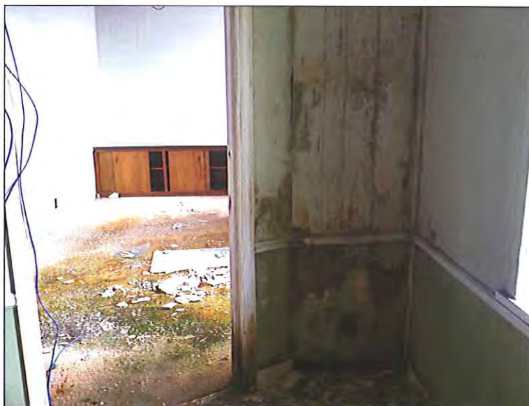
First Floor - West location - Moisture related staining/damage and microbial growth on wooden wall paneling and carpet
