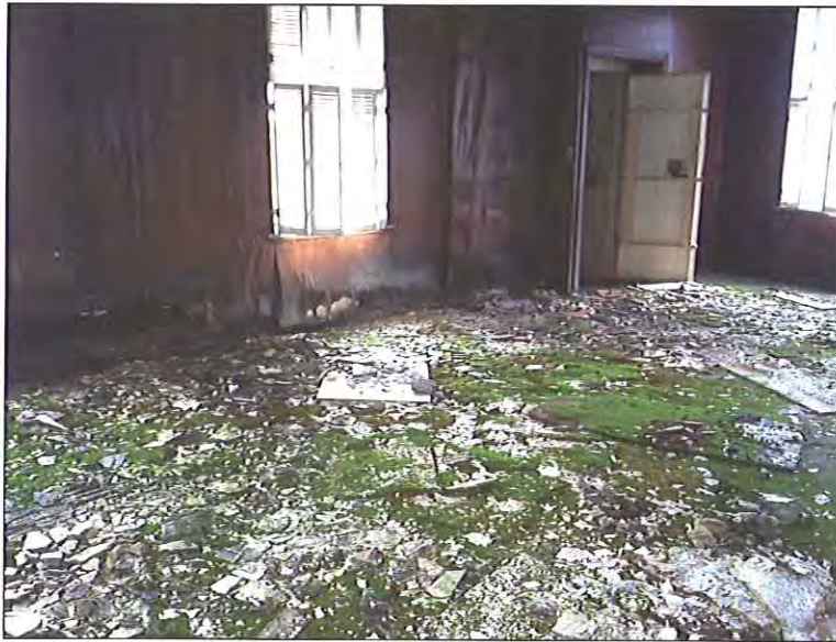
Fifth Floor - West location - Visible microbial growth as well as moisture related staining/damage on multiple building materials and contents
