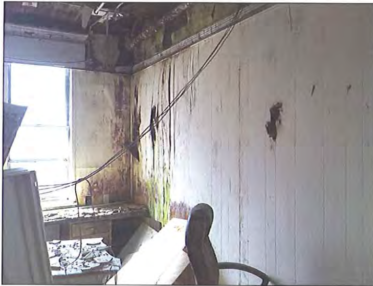
Fourth Floor - Southwest location - Visible mold growth with moisture related staining/damage on multiple building materials and contents
