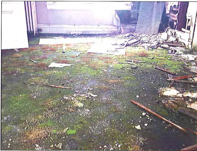
Fifth Floor - Southwest location - Visible microbial growth as well as moisture related staining/damage on multiple building materials and contents
