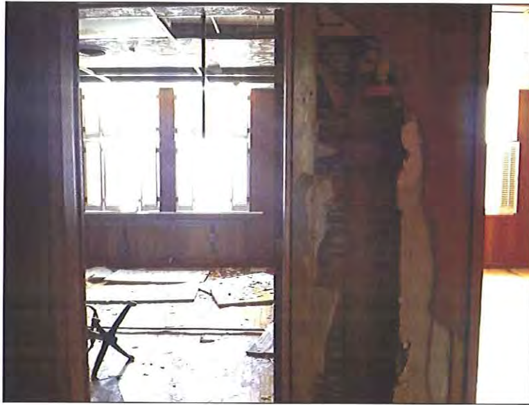
Second Floor - East location - Damaged ceiling and wall building materials
