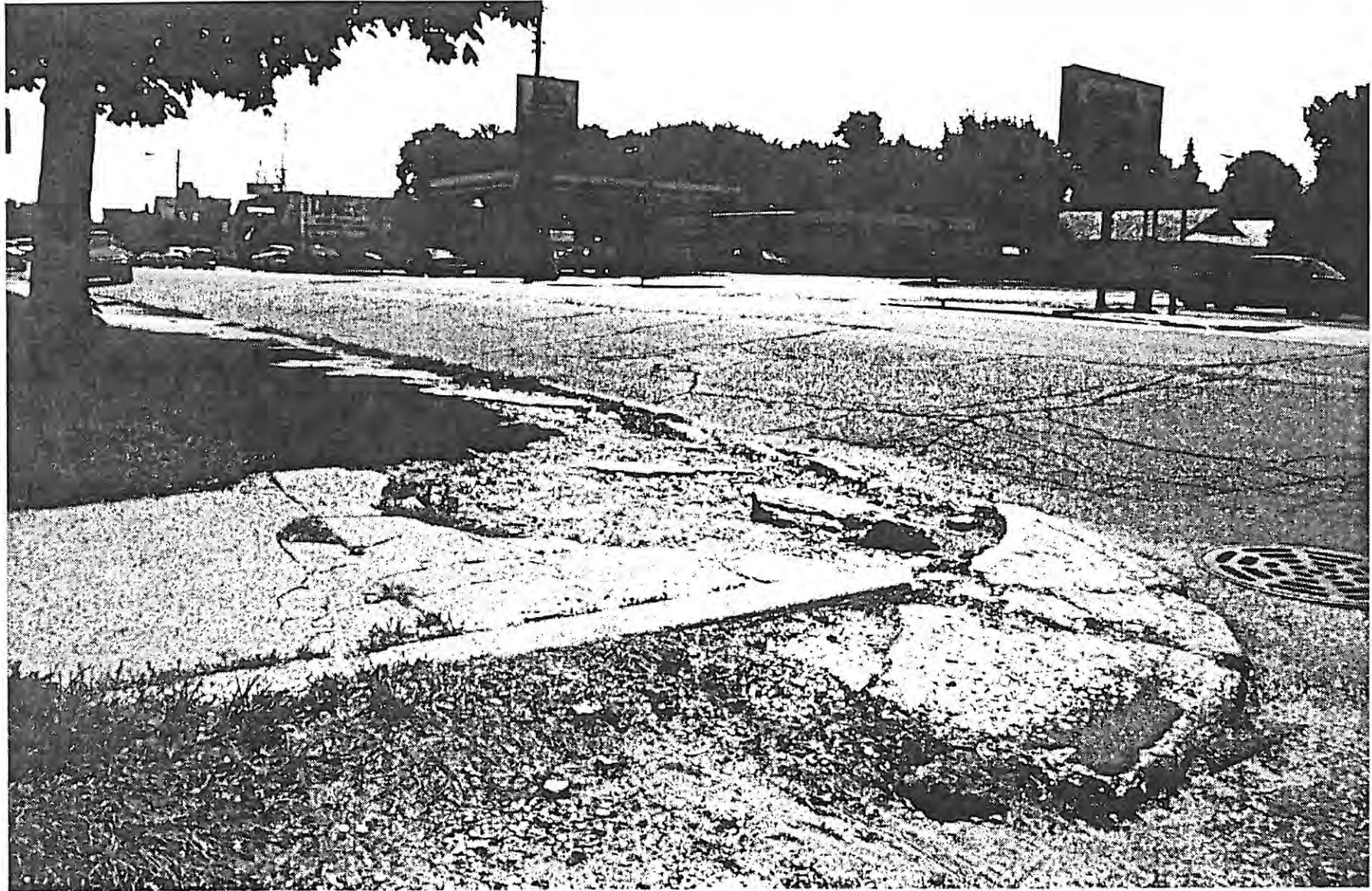
Sidewalks and crossings which are not passable by persons with disabilities, or even by children on bicycles or being pushed in strollers, pose serious threats to the safety of residents and visitors of all ages.
