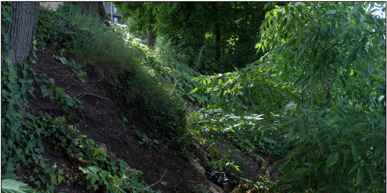
Bank erosion at Plaza Park
