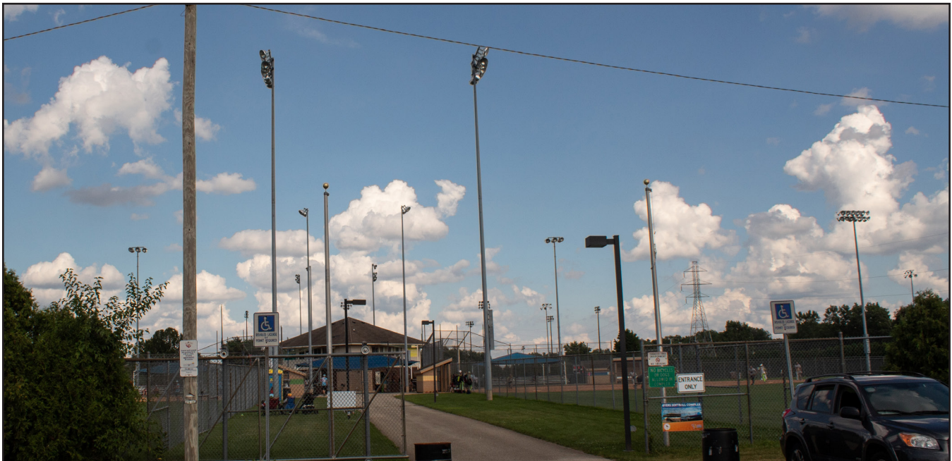
A plethora of outdoor lighting fixtures at the Byers Softball Complex
