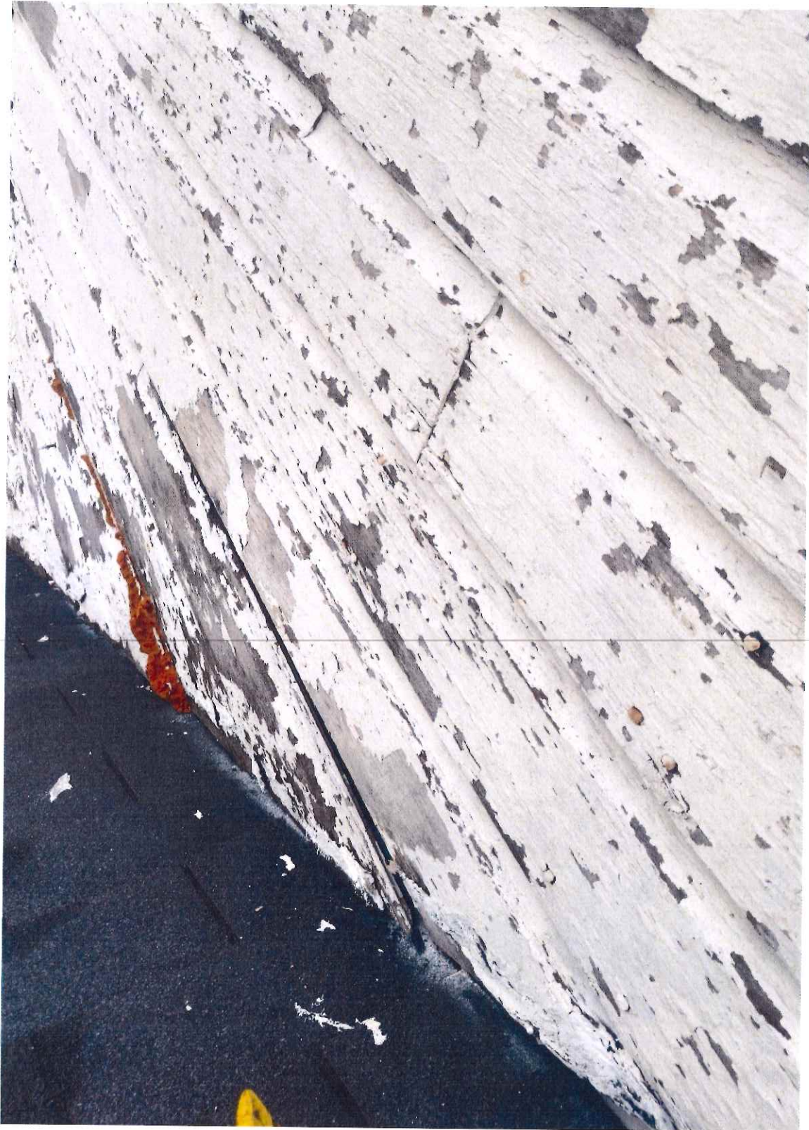
View of typical water entry point and deteriorated siding.
