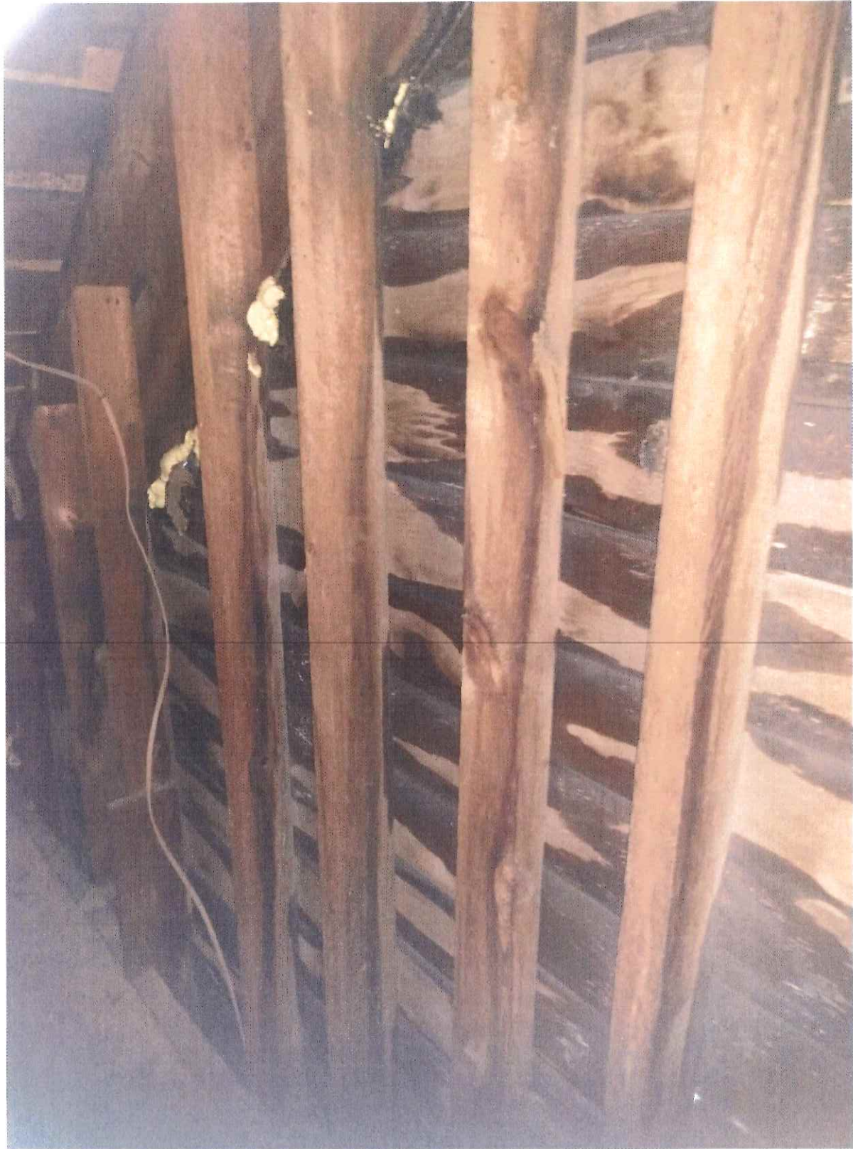
Soaked siding during rain event.
