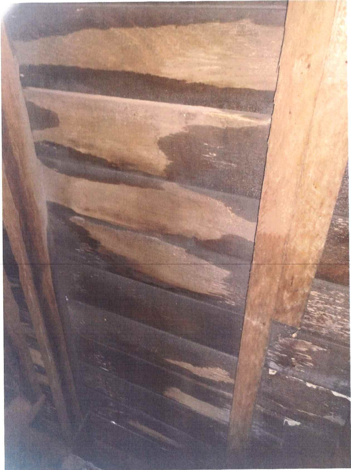
View of siding soaked during rain event (gable end of attic).
