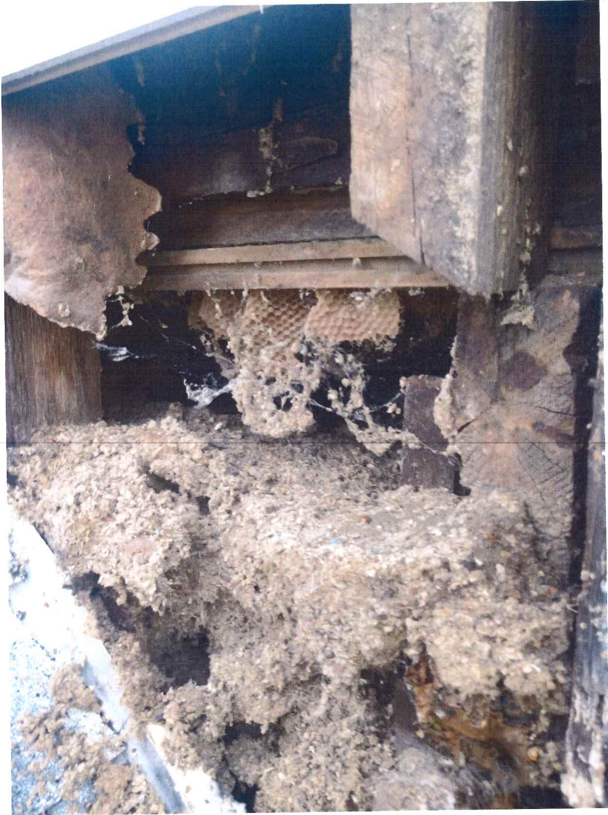
View of beehive, waterlogged floor joist, and waterlogged insulation in wall cavity.
