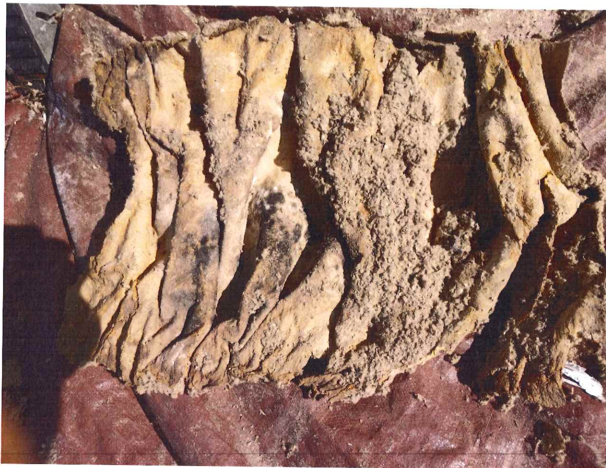
Moldy materials in wall cavities.
