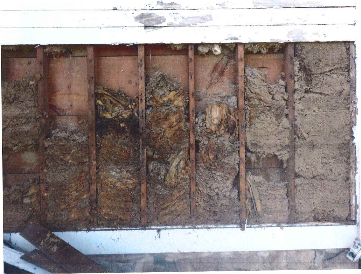
View of wet and moldy insulation/vapor barrier. Including bee hive and various animal feces.
