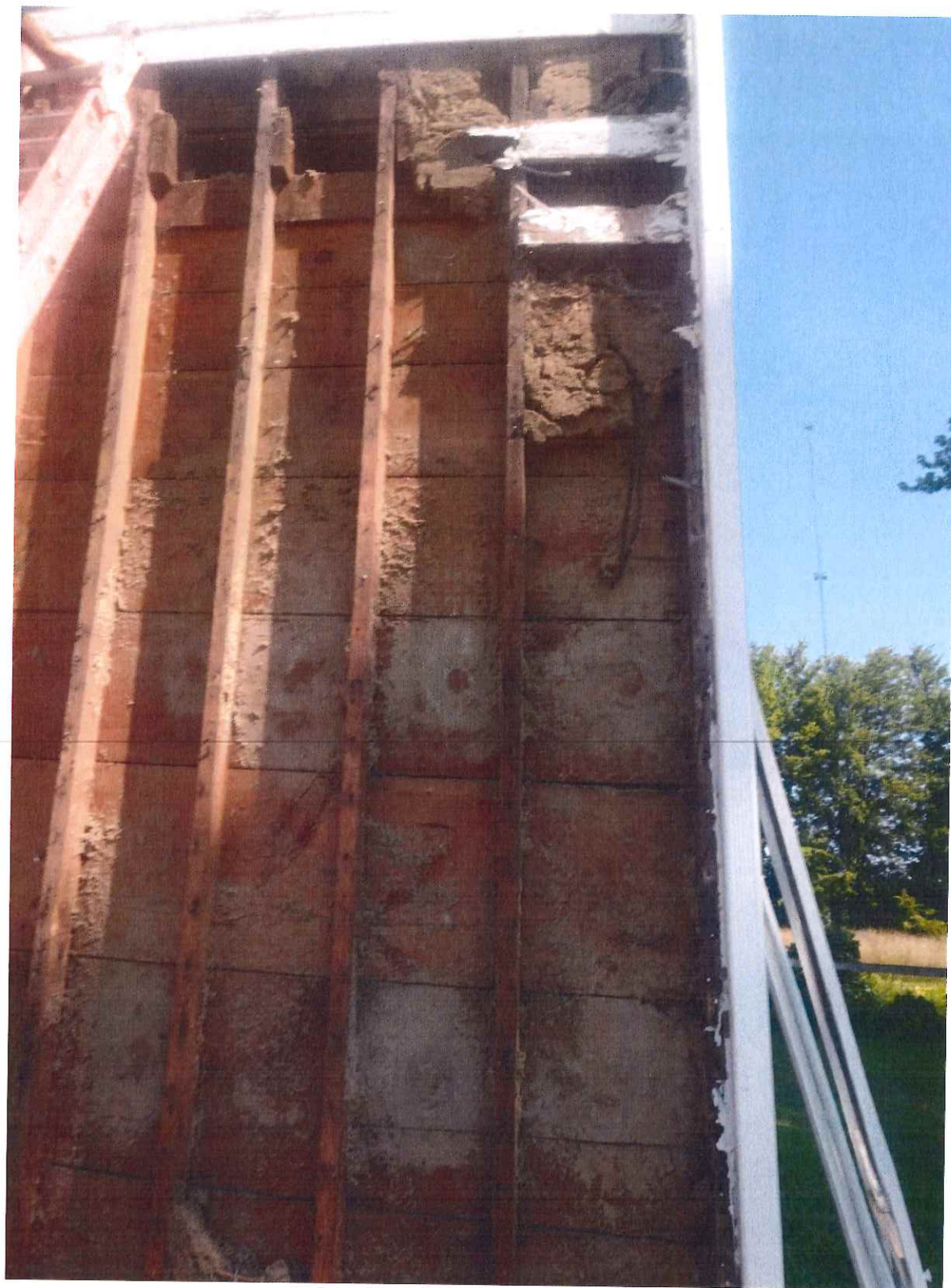
View of exposed wall and subsiding. This shows the only weatherproofing to the exterior wall cavity is the deteriorated wood siding.
