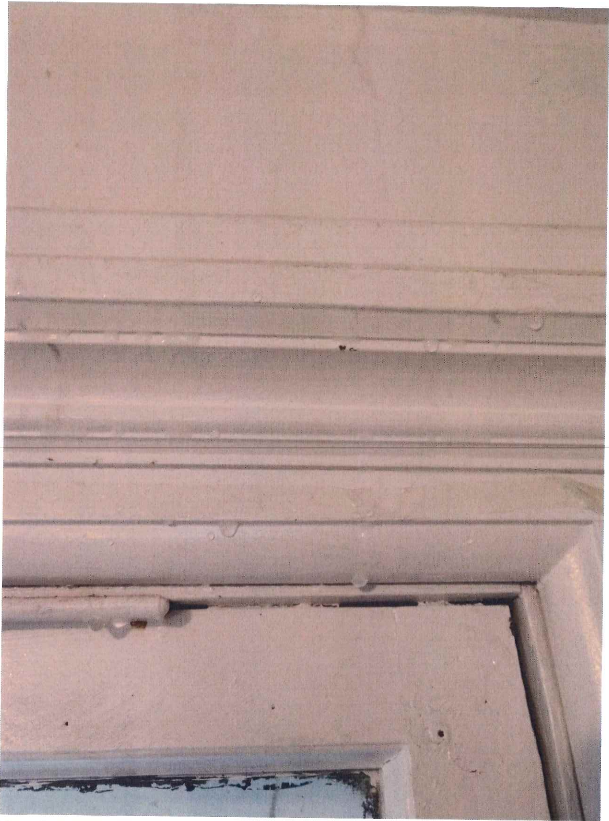
View of active water penetration above transom.
