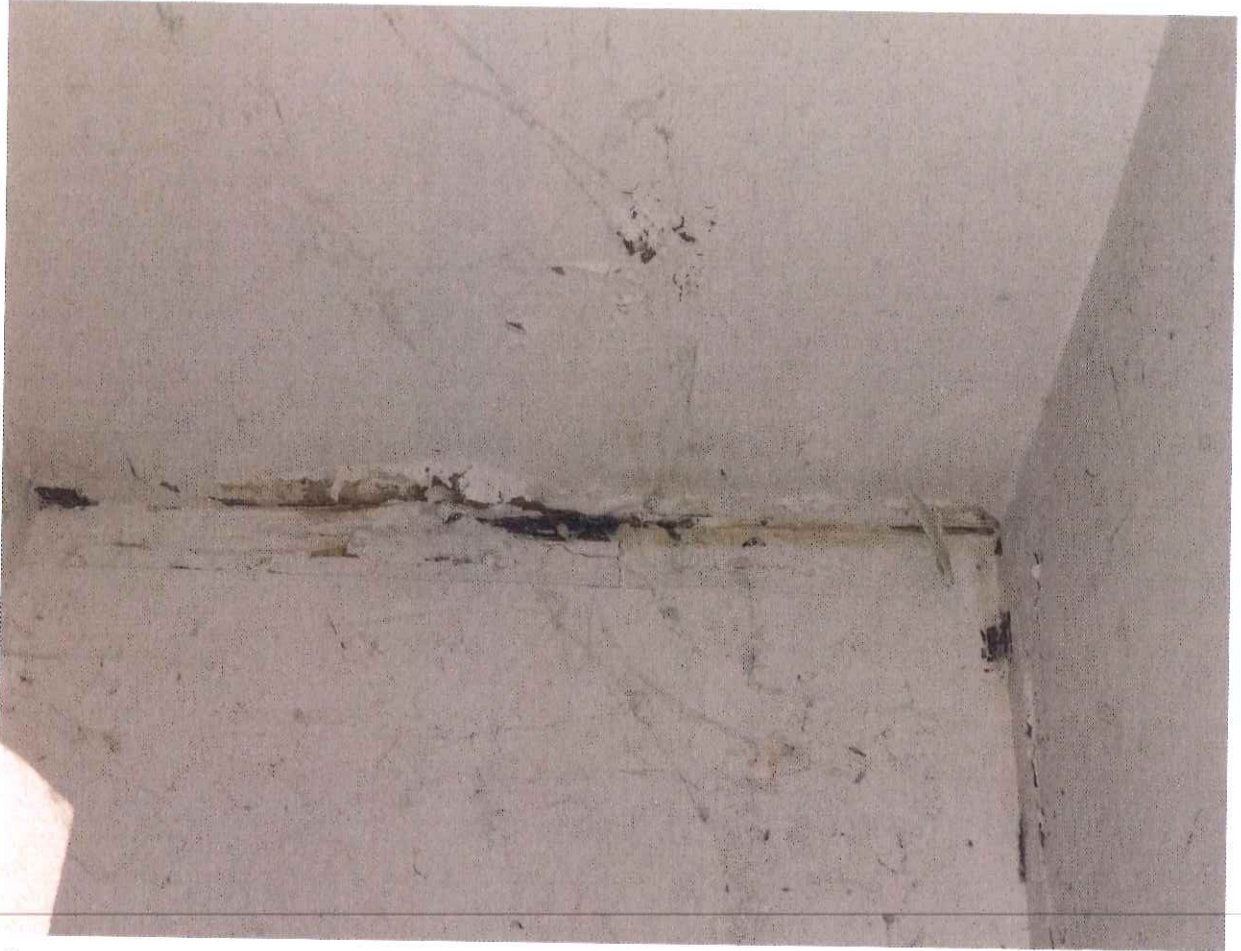
View of resulting water damage and mold in stairwell to the basement.
