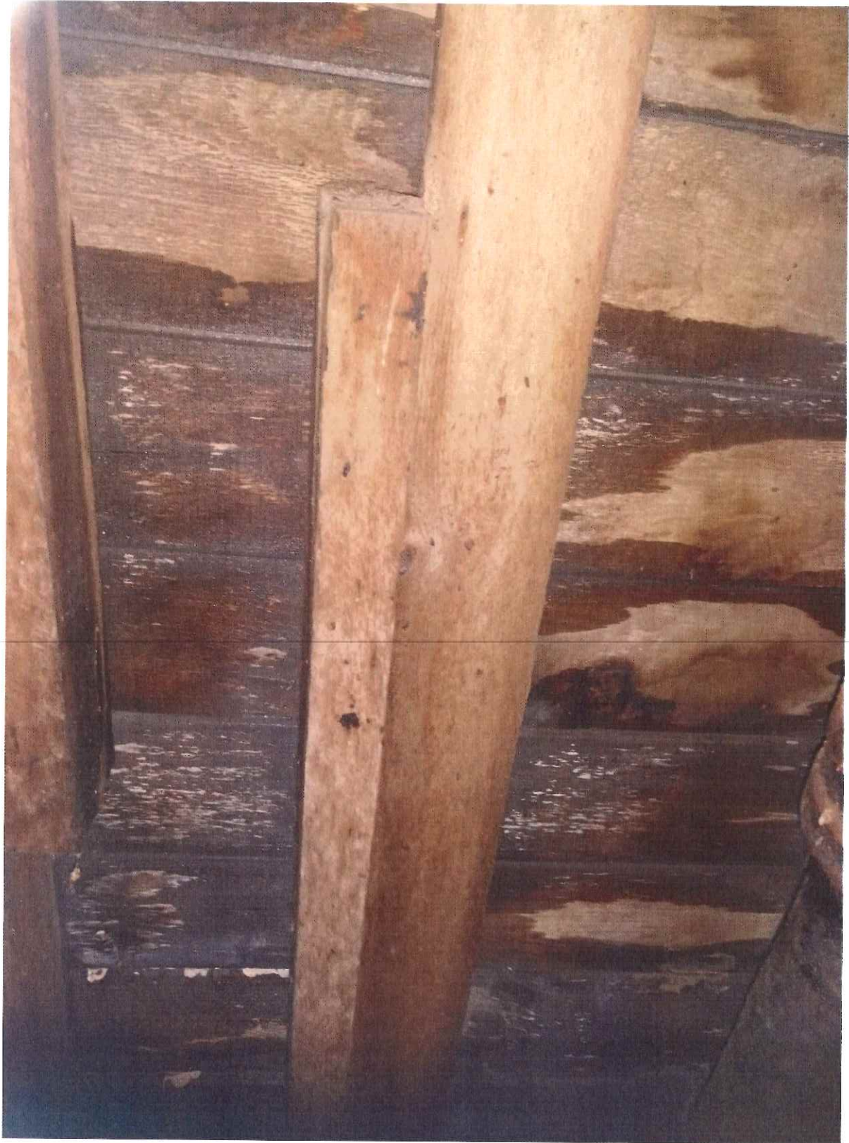
Soaked siding during rain event.
