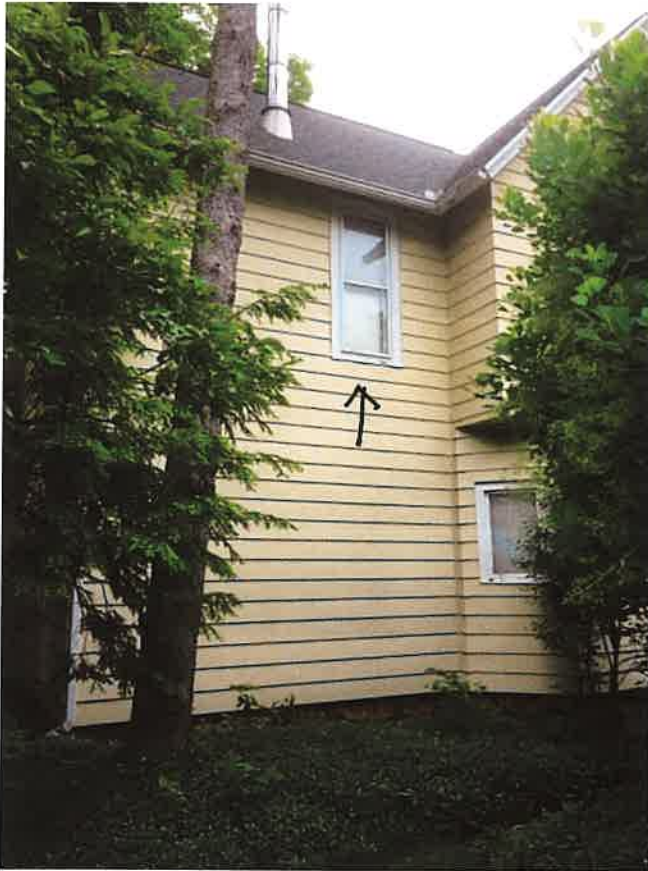
Figure 1. Near view of house showing window to be replaced.
