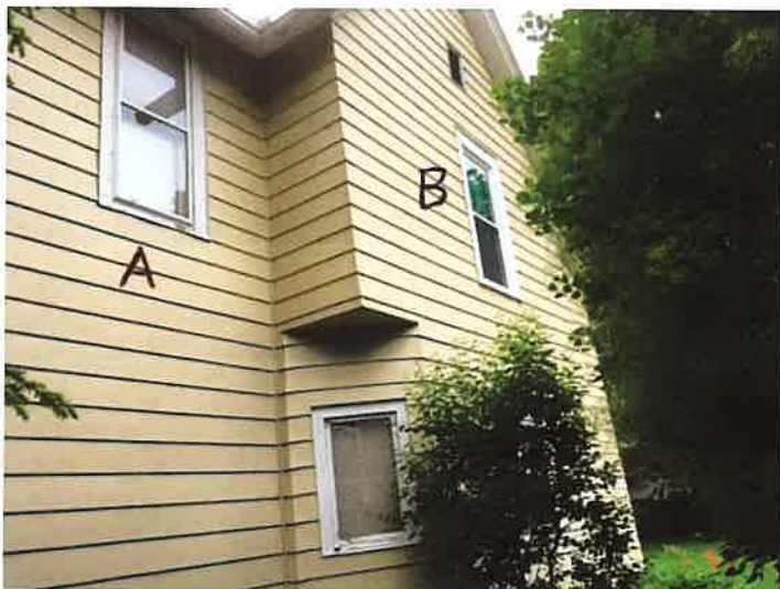
Figure 2. View of house, looking east, showing window to be replaced (A), and window replaced on 4/8/19 (B)
