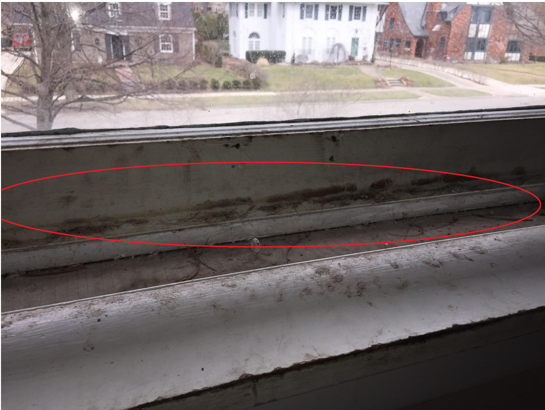
"Inside moisture damage"
