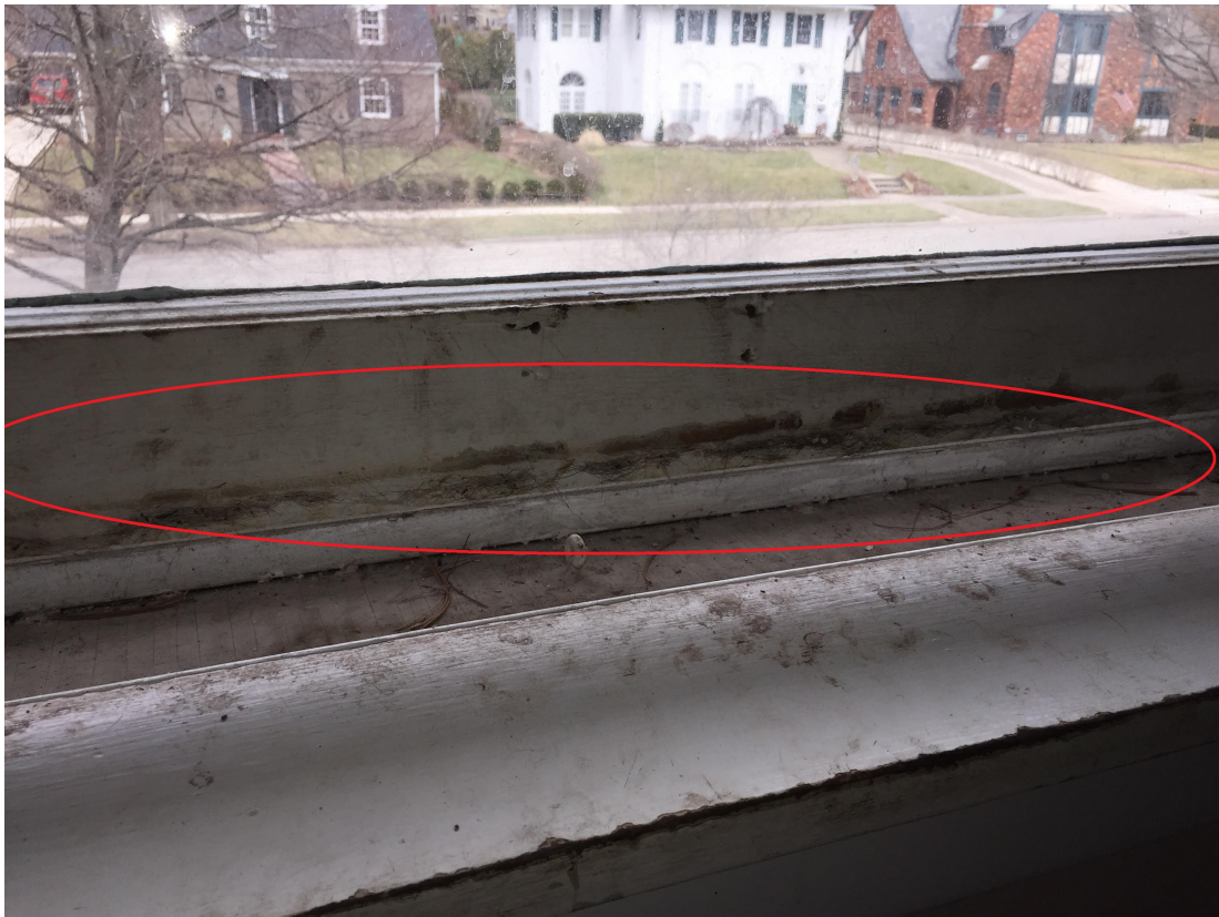
"Inside moisture damage"
