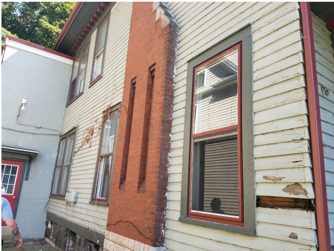
Figure 2 - North face, all windows to be replaced. – Photos from September.
