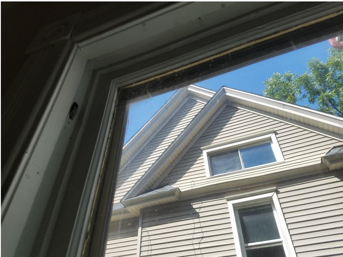
Figure 4 - Missing weights / ropes. – Photos from September.
