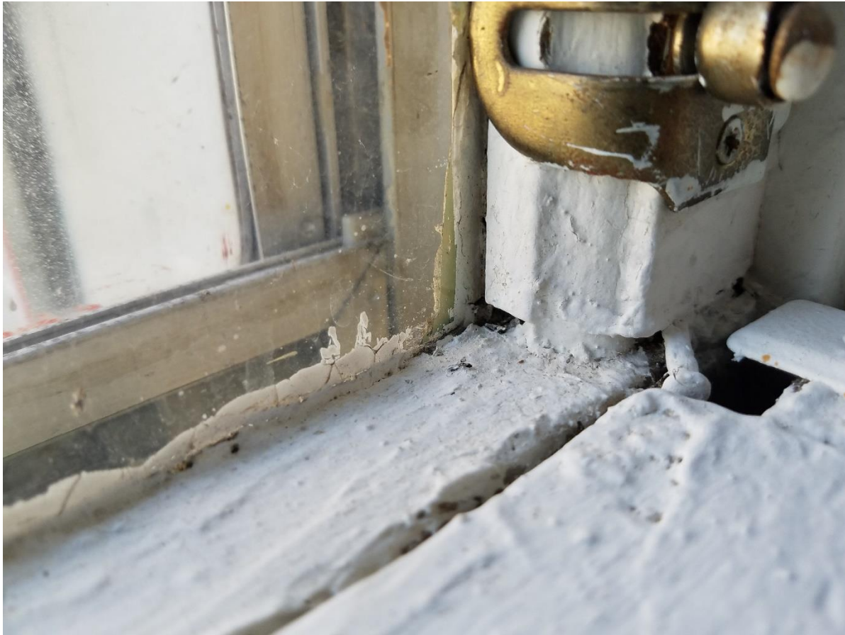
Figure 5 - Lower level window sash, nailed shut. – Photos from September.
