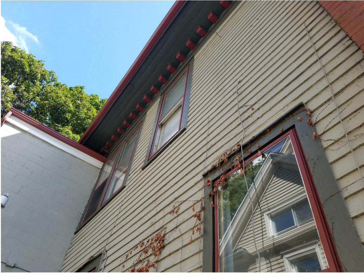
Figure 1 - North face, upper three windows to be replaced. – Photos from September.
